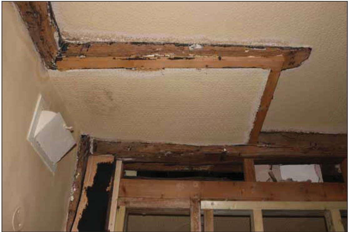
Plate 9 Downstand in GF01 in Building 1, taken from the east (DP 36)
