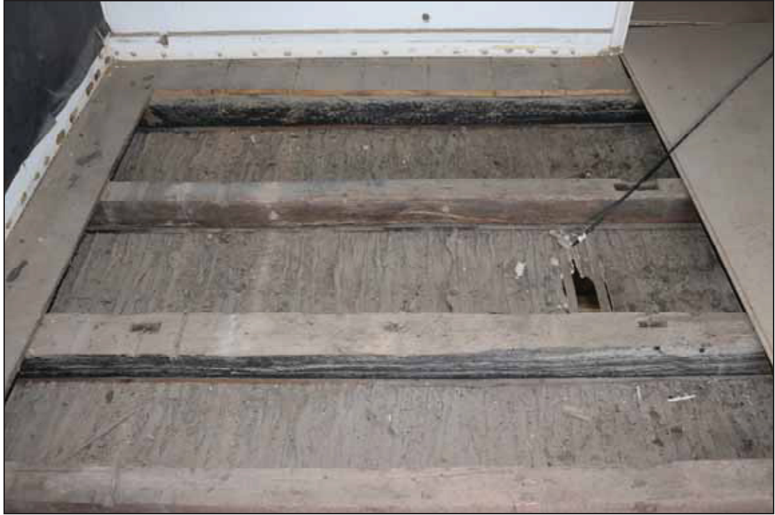
Plate 15 Exposed floor joists in FF01 in Building 1, taken from the south (DP 61)
