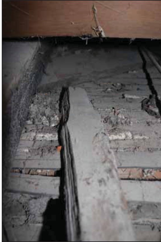
Plate 25 Area of exposed fabric along the rear of Building 1's historic core showing presence of wind braces, taken from the north (DP 58)
