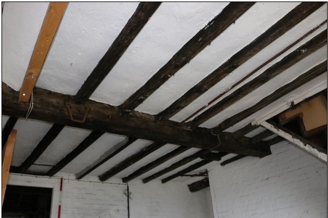
Plate 26 Detail of the ceiling joists in GF09, taken from the south (DP 097)
