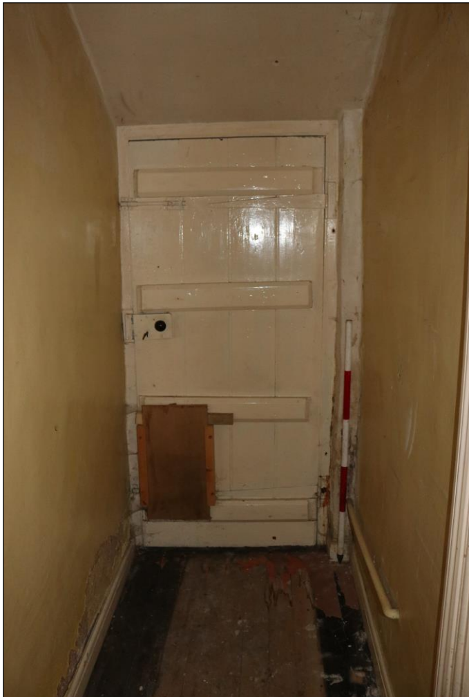
Plate 24 Boarded door in GF08 giving access to the rear yard, taken from the south-east (DP 051)
