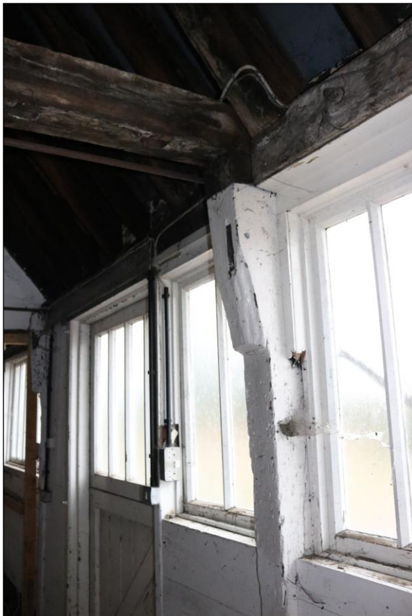
Plate 34 Detail of a jowled post to the bay division between GF10 and GF11, showing empty mortise for a downward brace, taken from the west (DP 106)
