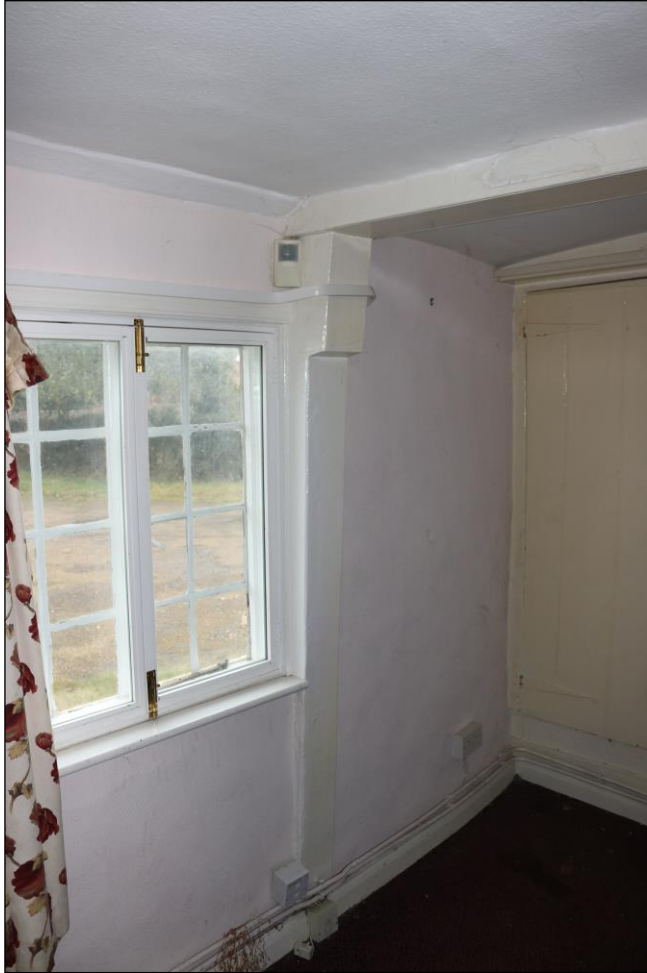
Plate 13 Splay-cut jowled post in GF02, with boxed-in binding joist above, taken from the north (DP 039)
