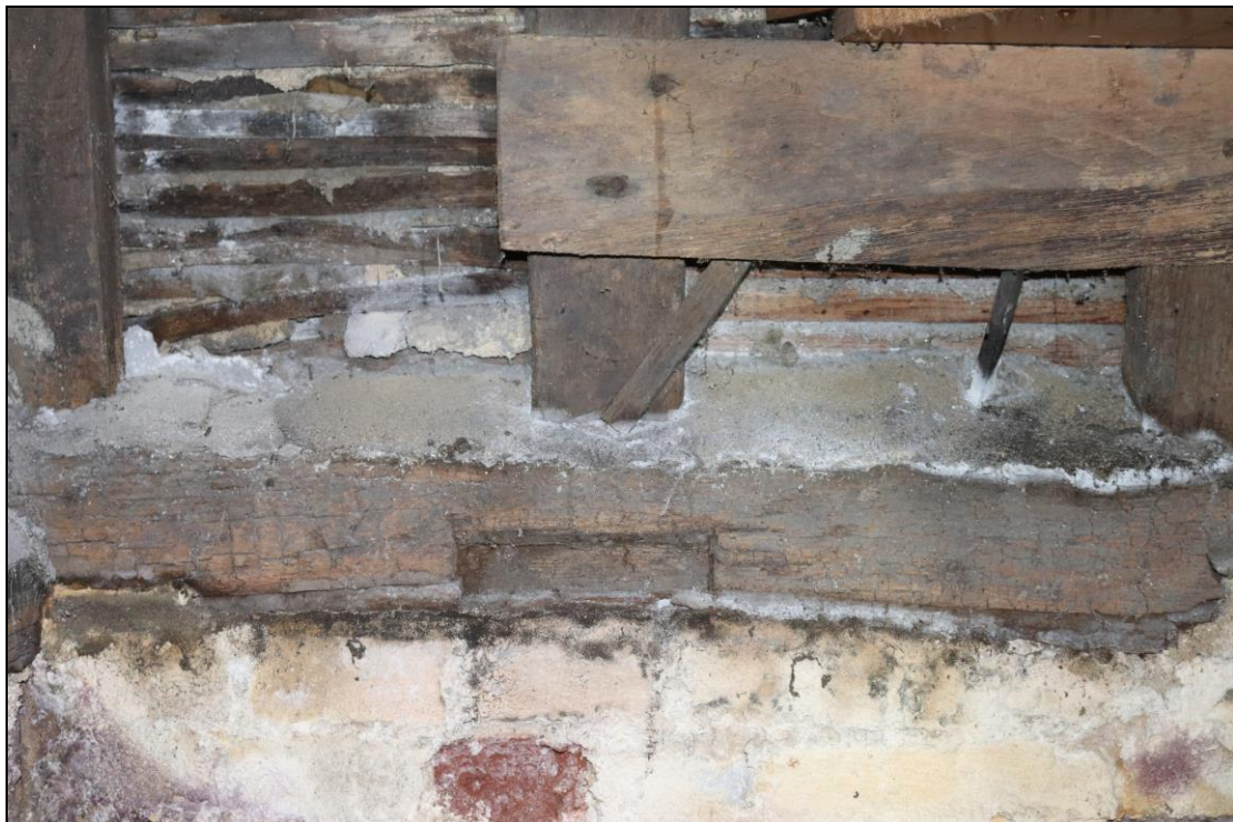
Plate 10 Exposed timbers in the under-stairs cupboard in GF01, showing brick sill and sole-plate with notch, taken from the south-east (DP 030)
