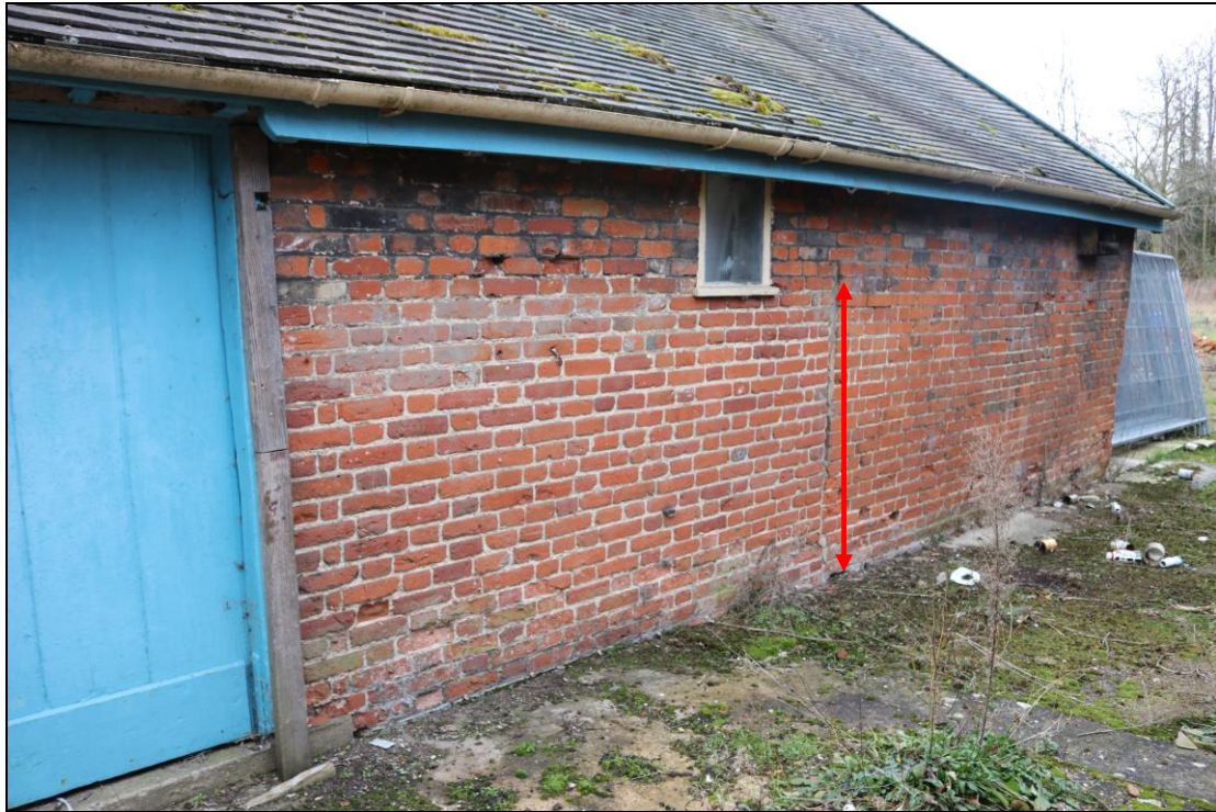
Plate 7 Rear wall of the Workshop, showing the straight joint in the brickwork (indicated), taken from the north-east (DP 013)
