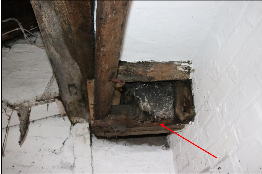
Plate 29 Detail of timber-framing in the area to the rear of GF09, showing some lath and plaster surviving (indicated), taken from the south-west (DP 116)
