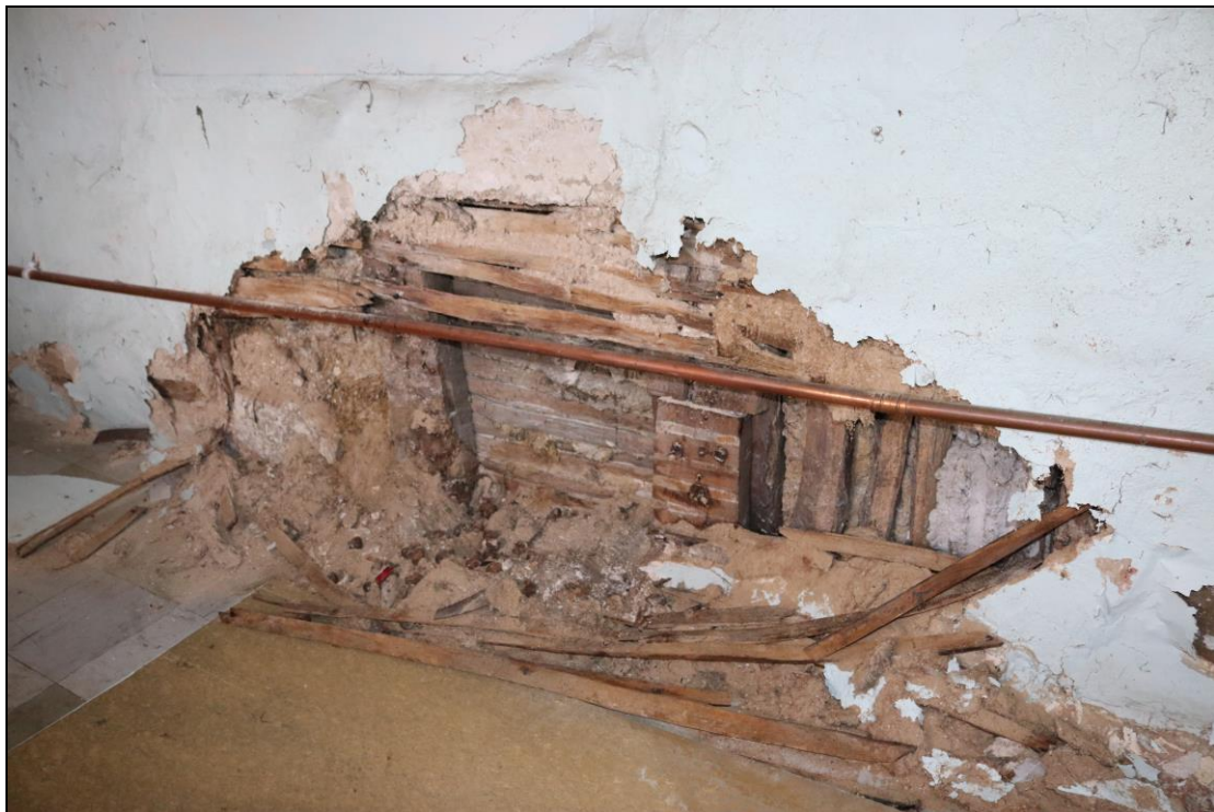
Plate 18 Detail of exposed timber-framing and phases of infill in GF04, taken from the north-west (DP 049)
