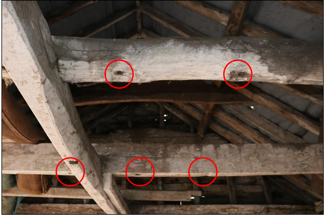
Plate 5 Roof structure over the Cartshed with detail of redundant peg holes (indicated), taken from the south-east (DP 122)
