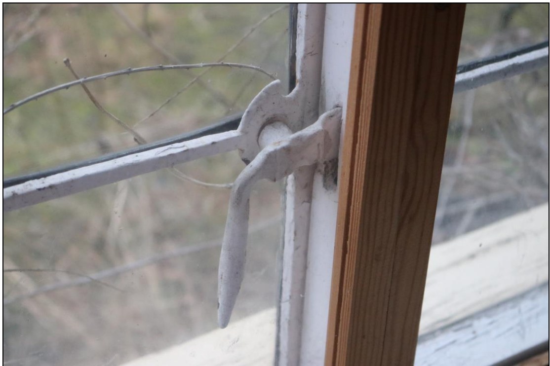
Plate 20 Detail of window catch in GF05, similar to many seen on the ground floor, taken from the north-west (DP 036)
