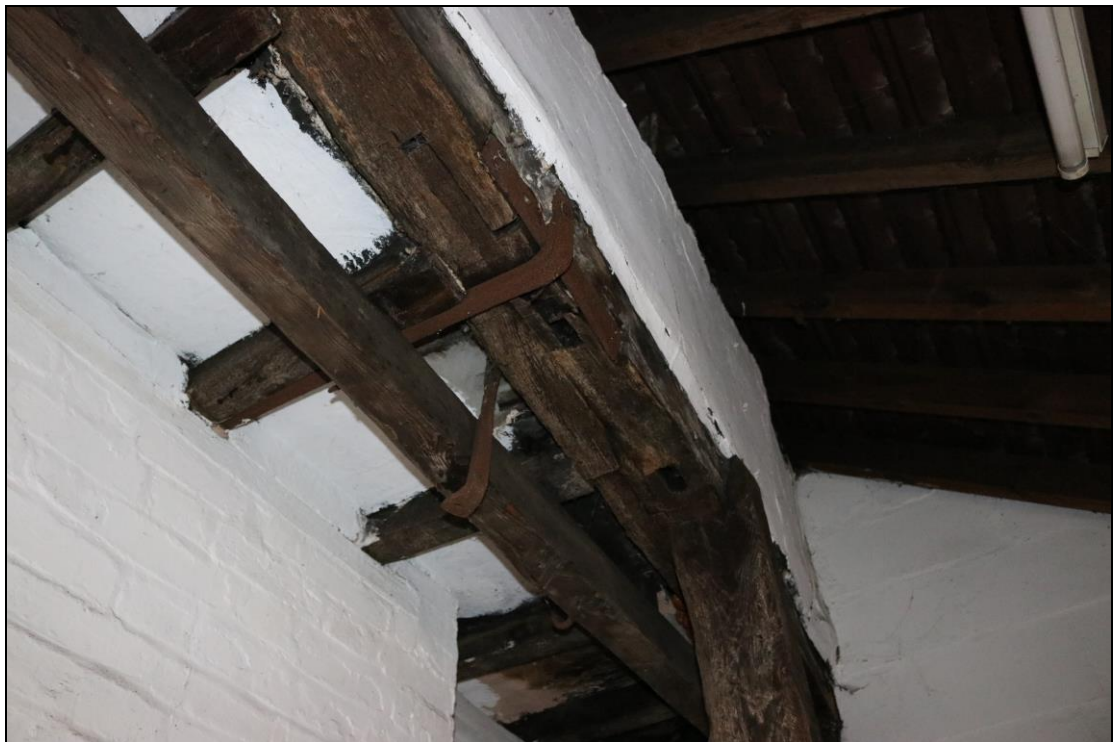
Plate 28 Detail of timber-framing in the area to the rear of GF09, taken from the north-east (DP 117)
