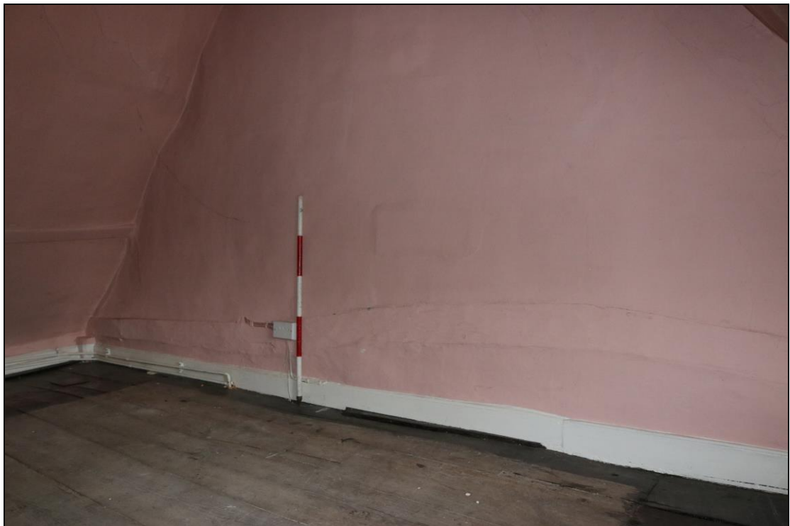
Plate 42 Interior of FF02, showing partially visible timber-framed elements, taken from the south-west (DP 075)
