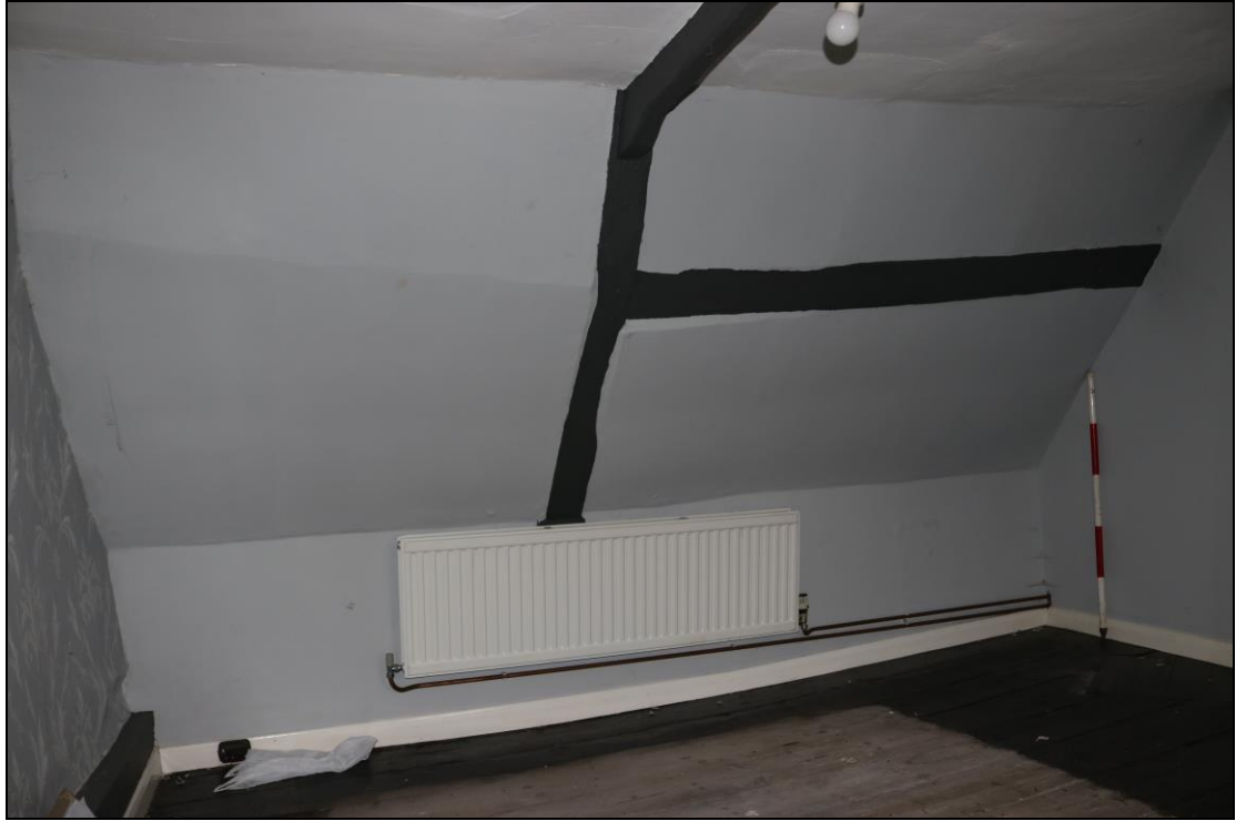
Plate 45 Interior of FF04, showing partially visible timber-framed elements, taken from the south-east (DP 063)
