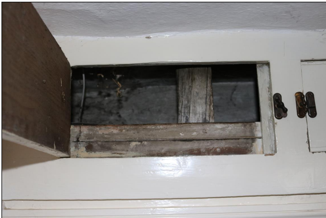
Plate 12 Detail of exposed timber including stud and horizontal, within a cupboard in GF02, taken from the south-west (DP 038)
