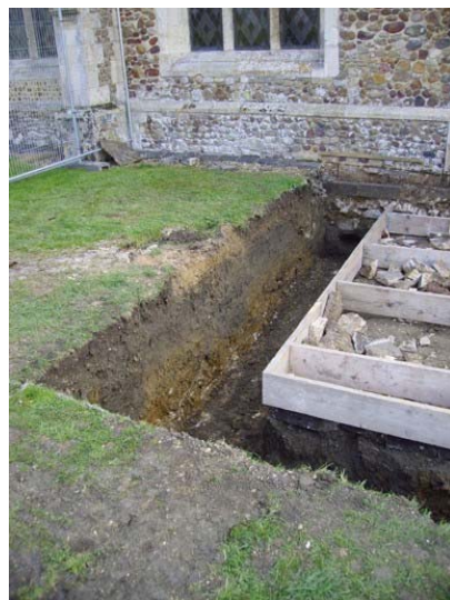
DP 6. Oblique shot of Section 2. Timber shuttering negated a square on photo, view SE
