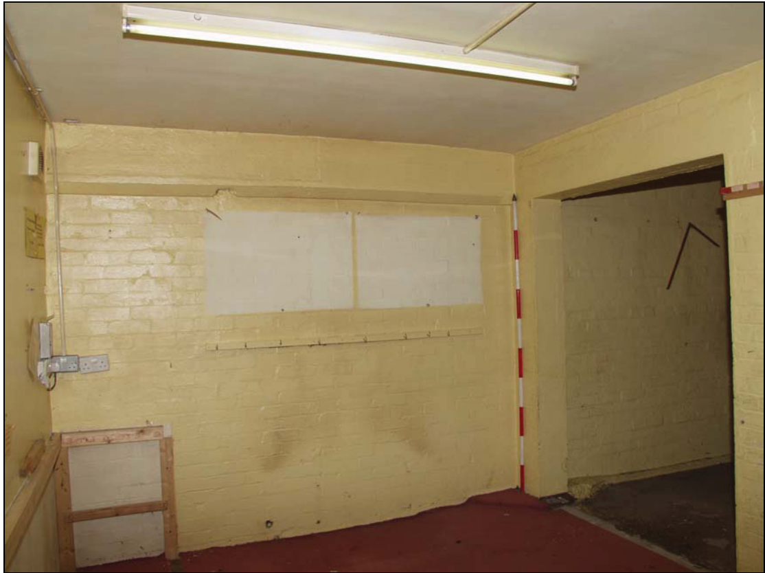
Plate 11 Blocked aperture on west wall of Unit 7, Building Group 3, taken from the south-east (DP 55)
