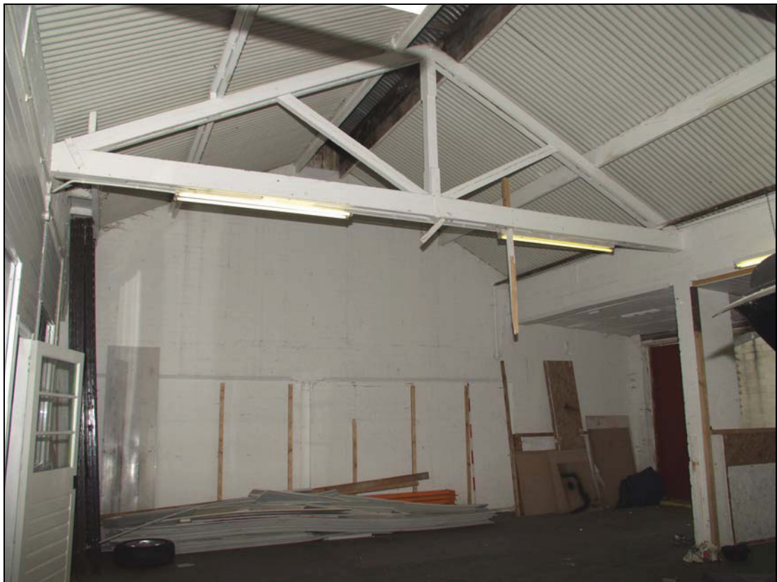
Plate 12 Blocked apertures at the west end of Unit 8, Building Group 3, taken from the south-east (DP 65)
