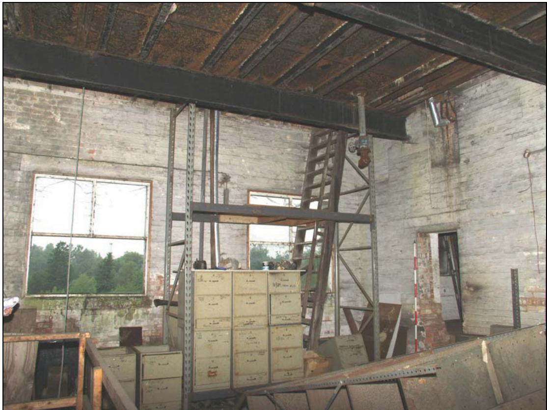
Plate 5 Room 4, Building 2 showing stair to upper floor, taken from the south-west (DP 10)
