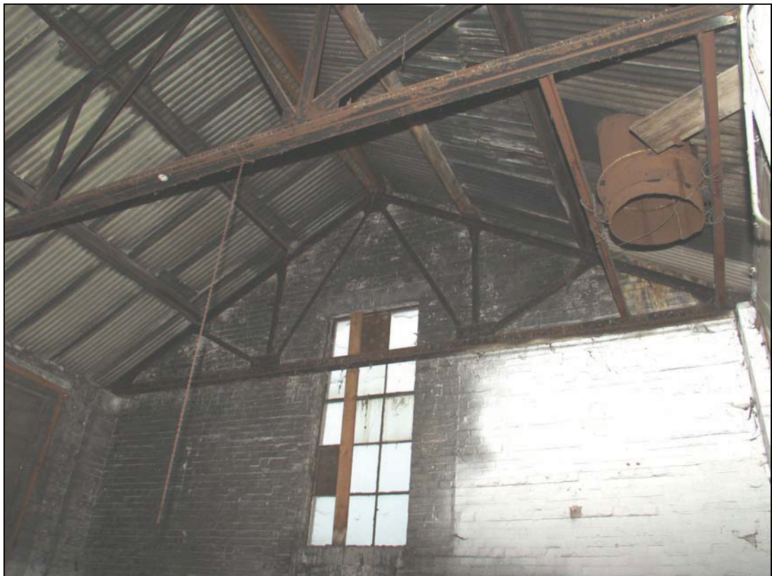
Plate 4 Room 2, Building 2 showing remnant of chimney flue from coal fired boiler, taken from the south-west (DP 6)
