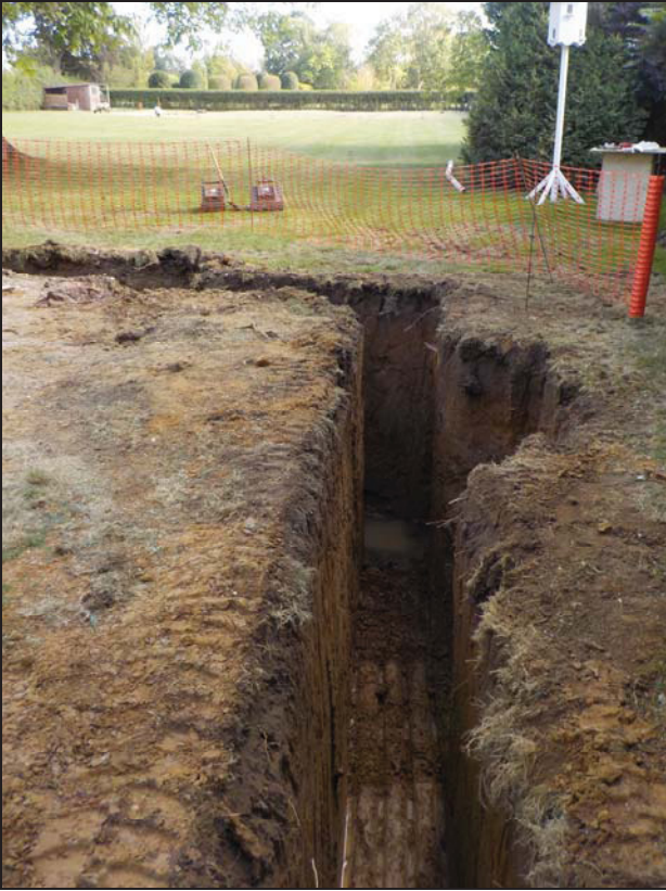
7 View of the trench showing depth of sample section 2 in the corner
