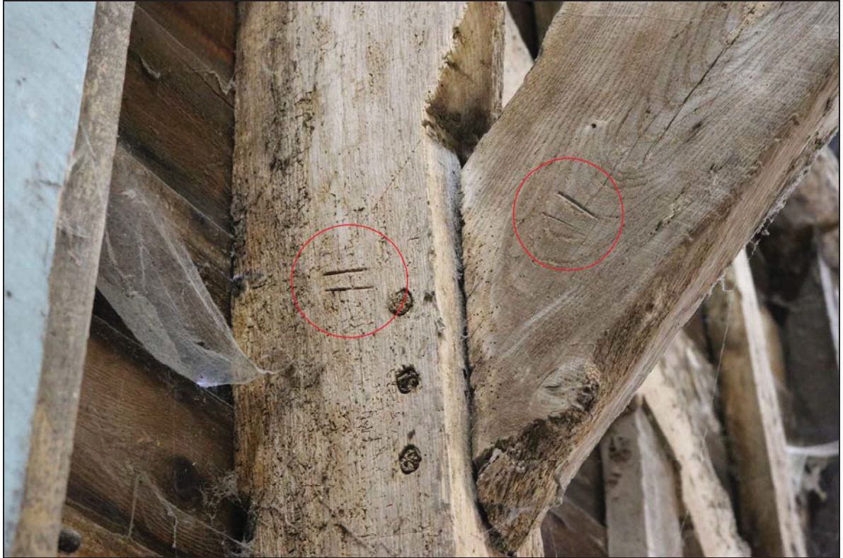
Plate 7 Detail of the carpentry marks and three pegs on the brace and post of Bay 3, taken from the east. (DP 34)
