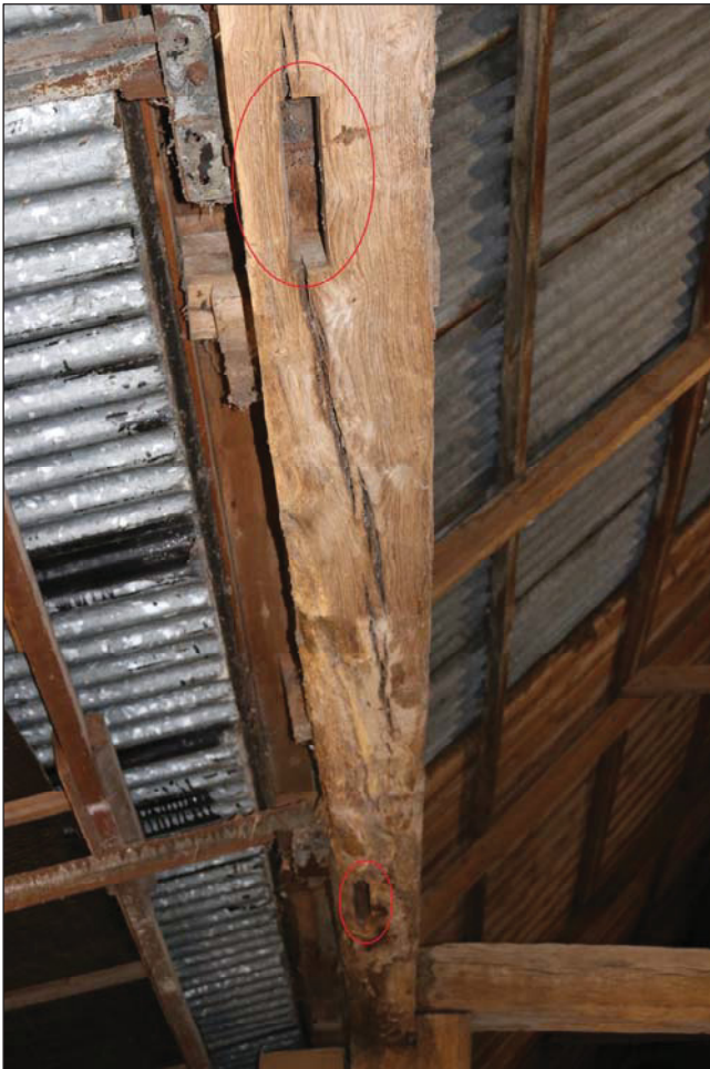
Plate 5 Detail of the wall plate, highlighting the empty mortices for braces, taken from the north-west. (DP 32)
