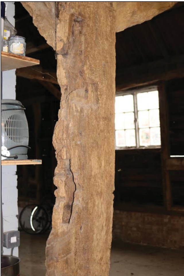
Plate 6 Detail of empty post mortice, evidencing former aisle, taken from the north. (DP 33)
