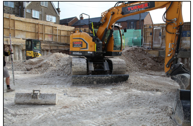
22 View of site looking north-east after the excavation of the new basement
