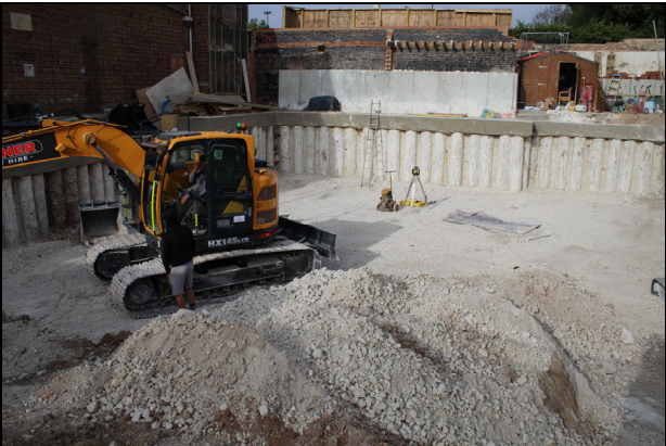
19 View of site looking west after the excavation of the new basement
