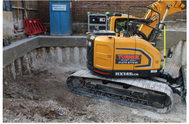
24 View of site looking south after the excavation of the new basement
