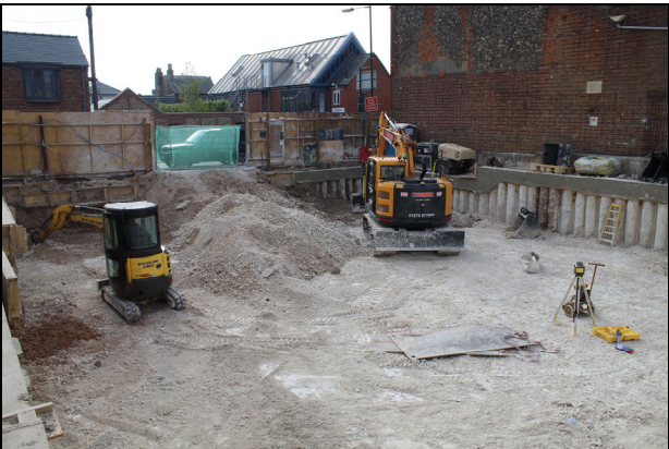
21 View of site looking south-east after the excavation of the new basement
