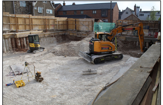
20 View of site looking east after the excavation of the new basement
