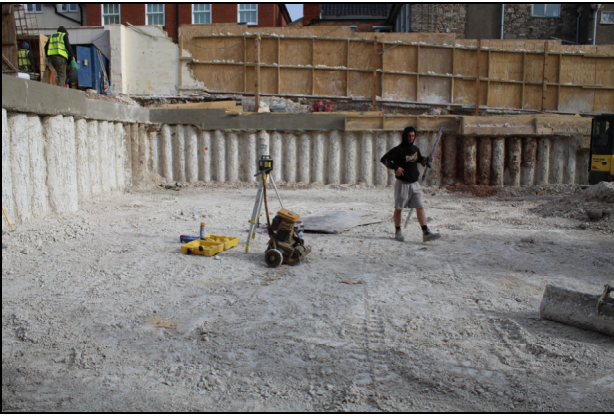
23 View of site looking east after the excavation of the new basement
