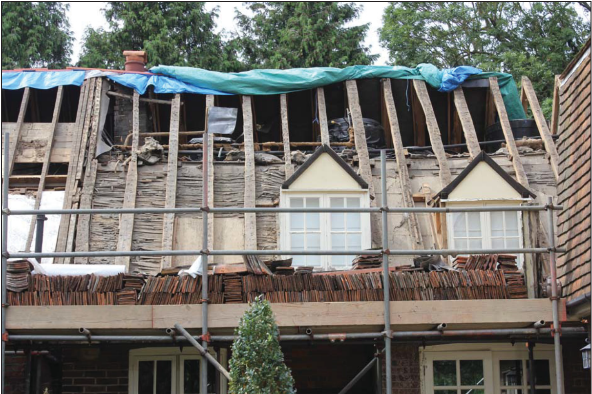
Plate 7 View of the east roof pitch of the historic core, taken from the east (DP 86)
