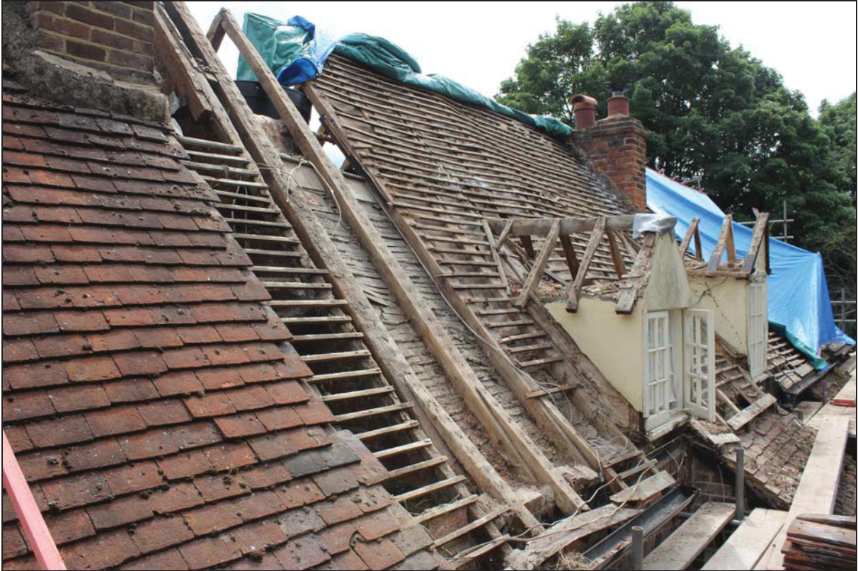
Plate 6 West roof pitch of the historic core showing exposed rafters and dormer windows, taken from the north-west (DP 47)
