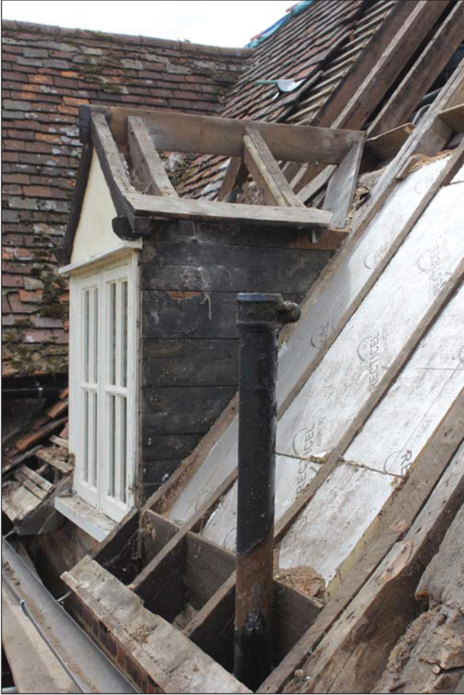
Plate 13 View of the east roof pitch of the historic core, taken from the east (DP 86)
