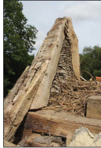
62 Detail of the dormer window (Range 1: Bay 2, west side) showing gable with steel mesh and cement render, taken from the south
