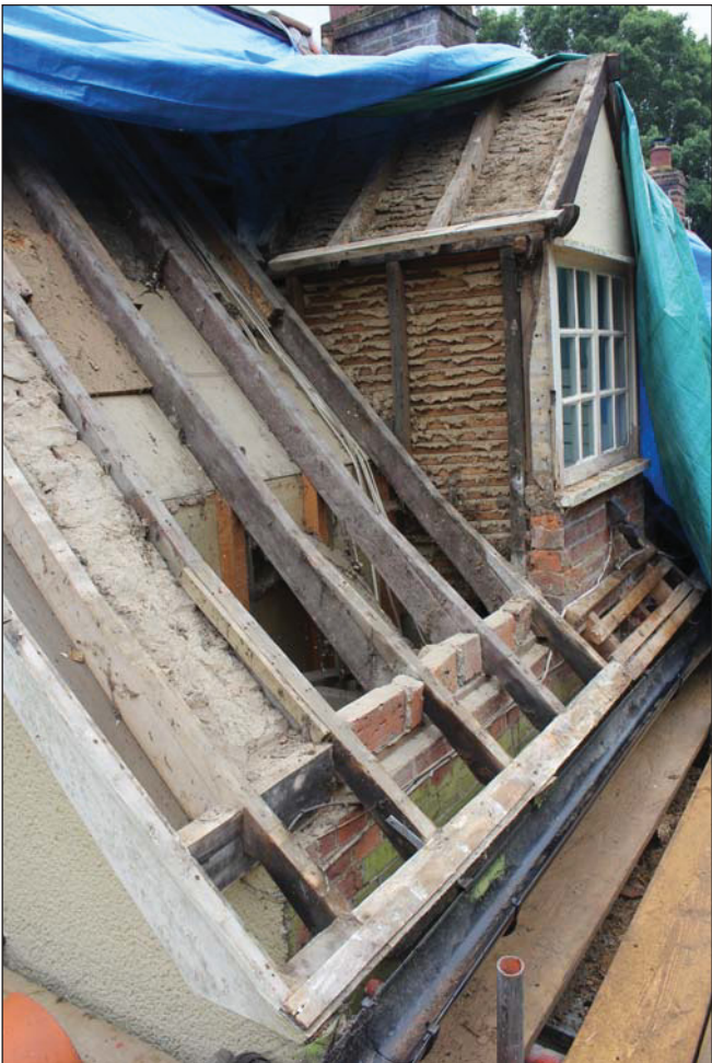
Plate 14 West roof pitch of Range 4 showing dormer window, taken from the north-east (DP 89)
