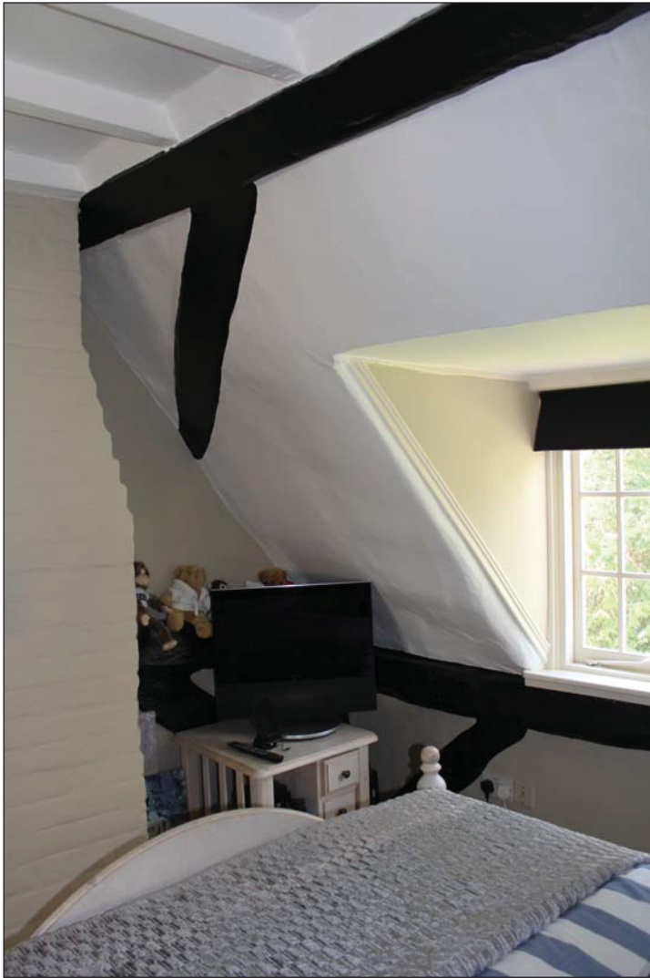
Plate 3 West side of Room FF07 showing exposed timber elements including a wind brace and lower inner brace, taken from the north-east (DP 24)
