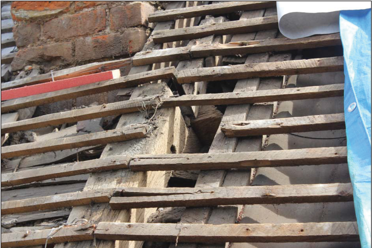
Plate 12 West roof pitch of the historic core (Bay 1: south end) showing principal rafter with pegged collar and weathered projecting purlin end, taken from the west (DP 67)
