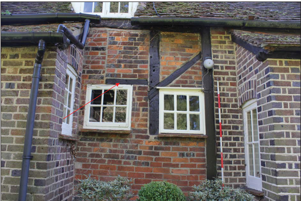
Plate 2 Section of the west elevation showing timber-framing infilled with brick and position of possible early window (indicated), taken from the west (DP 04)
