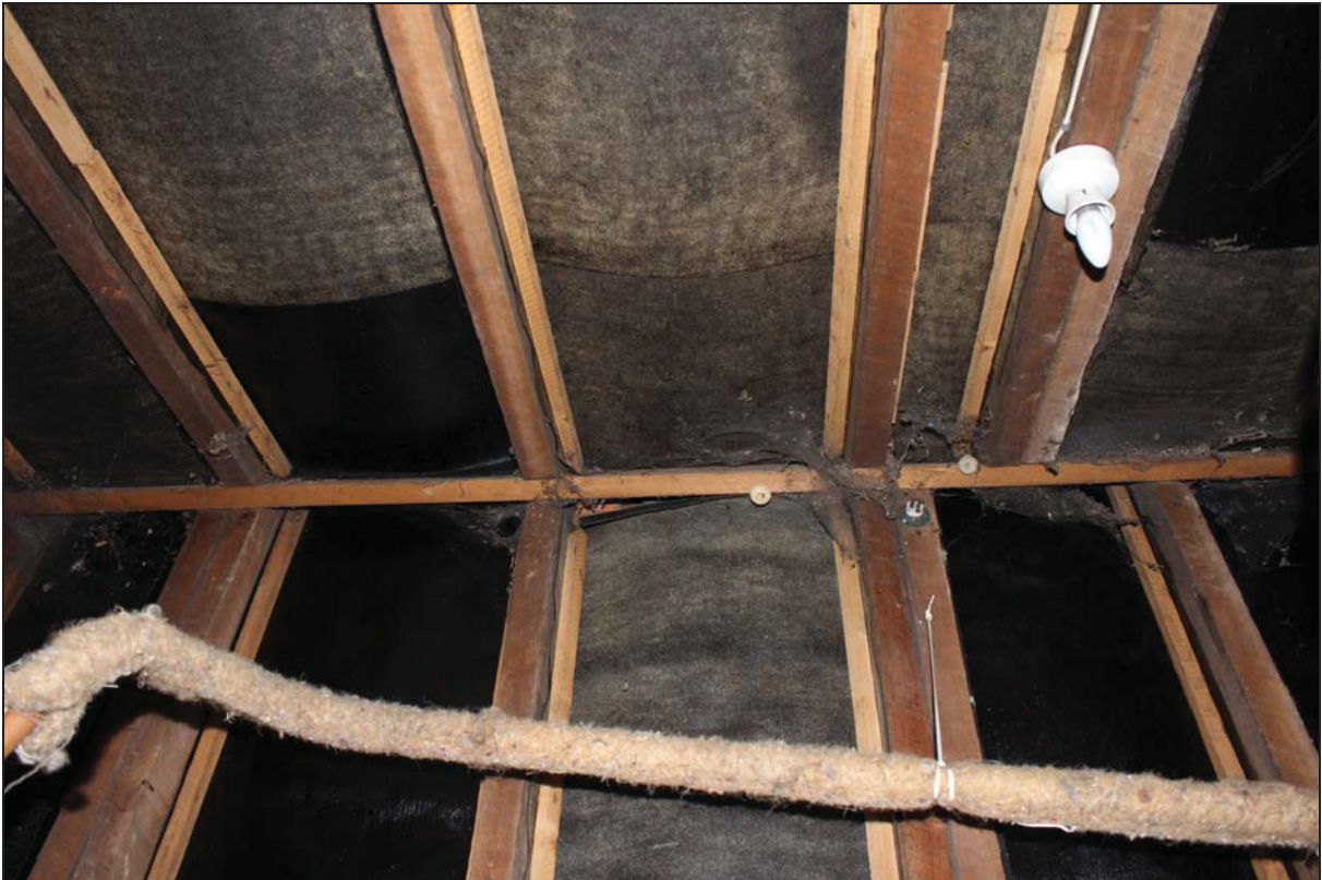
Plate 5 View of the roof apex in the south end of the main range, taken from the west (DP 14)
