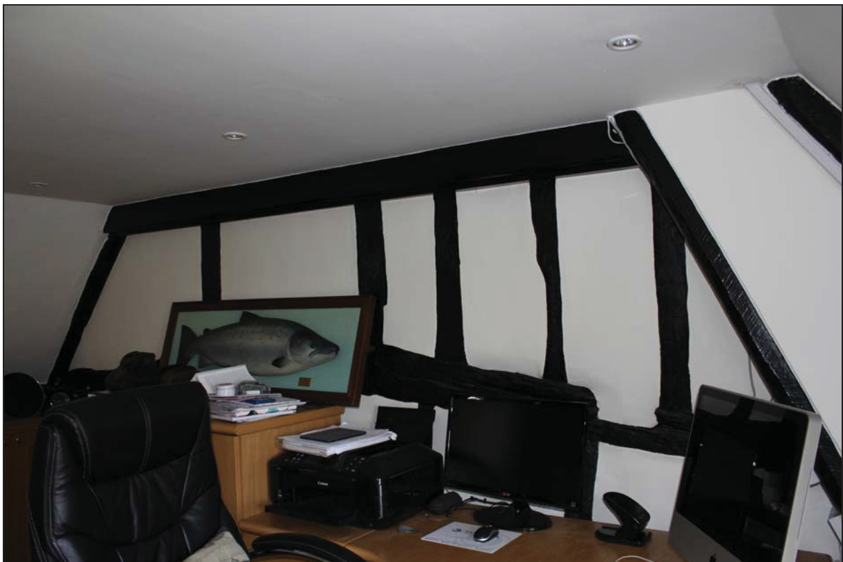
Plate 4 View of the south gable end of Range 1 exposed within Range 2 (FF08), taken from the south-east (DP 22)
