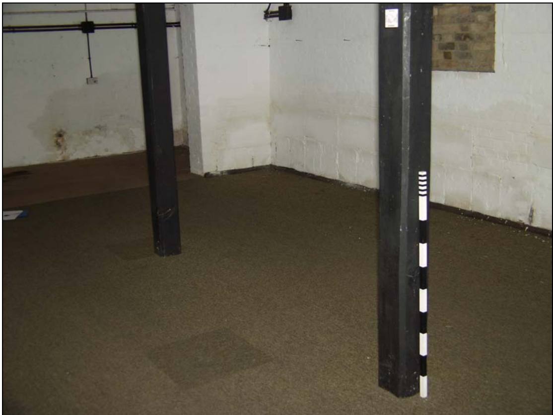
19 Wooden columns and slate damp proof course to ground floor of eastern section, taken from the south-east (32)
