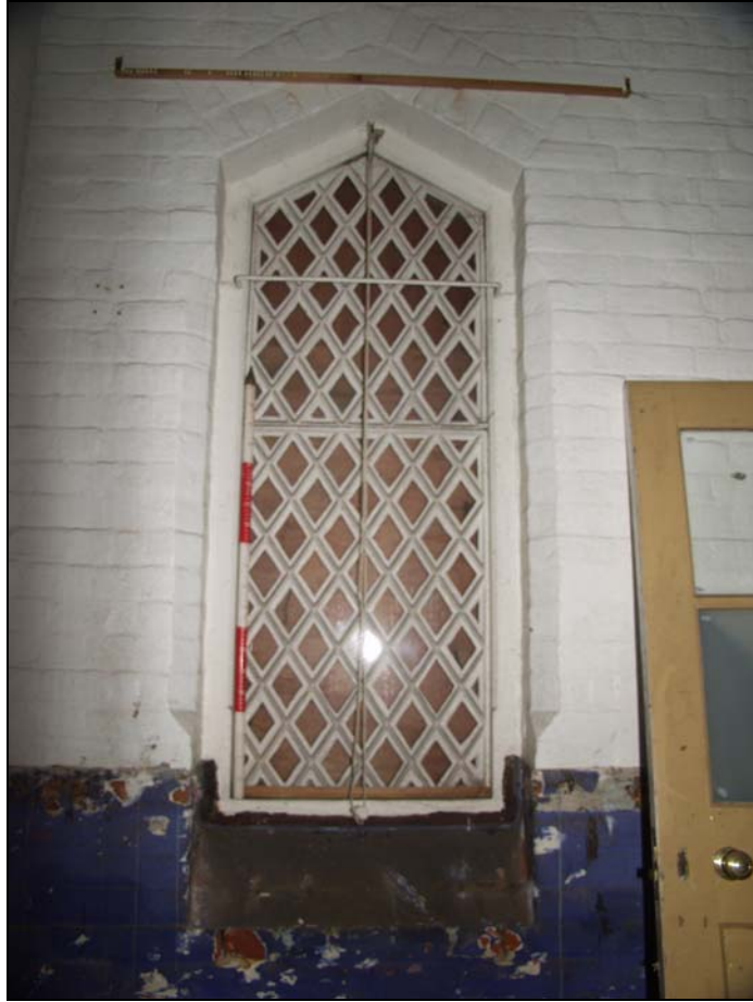
Plate 5 Gothic style window on the north wall of Room 4, taken from the south (33)
