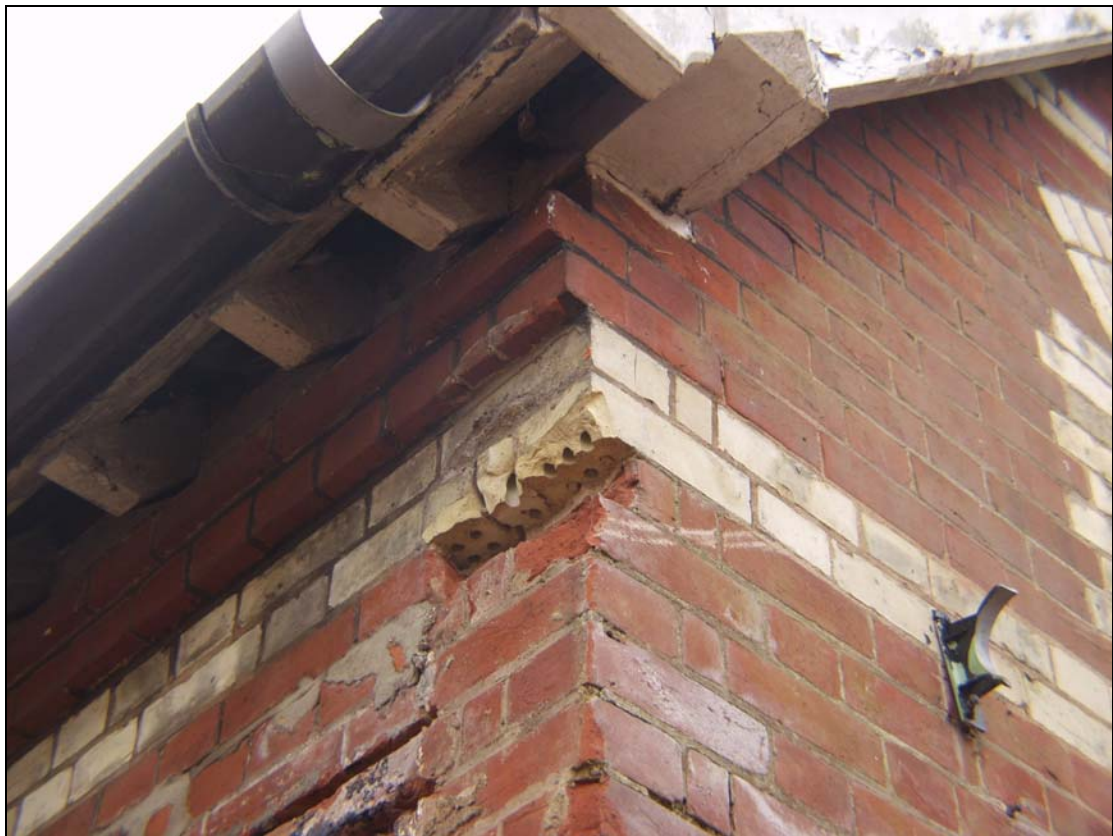
Plate 2 Brick banding on the rear range with typical Arlesey brick characteristics, taken from the north-east (20)
