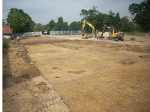
DP 2. General view of the site looking north, with the southern Phase 1 enclosure in the centre.
