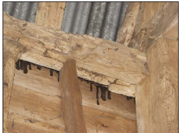
96 Face-halved and bladed scarf joint in the north wall-plate of Building 2 (Bay 4), taken from the south
