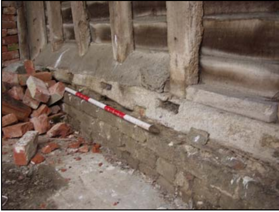
85 Redundant mortices in the north sill-beam of the porch (Building 1) for a raised floor, taken from the south-east
