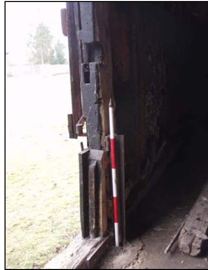
100 Detail of threshing leap socket on west side of doorway (Building 2), taken from the north-east
