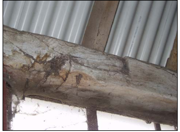
92 Simple scarf joint in the east wall-plate of Building 3, taken from the west
