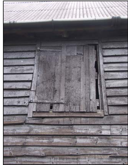
94 Detail of high-set loading door on south elevation of Building 2 (west end), taken from the south
