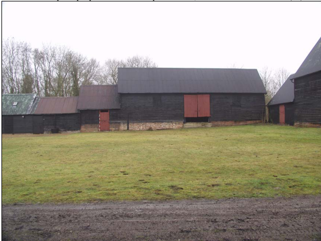
Plate 6 North range (east end) including Building 2 (timber-framed barn), taken from the south (5)
