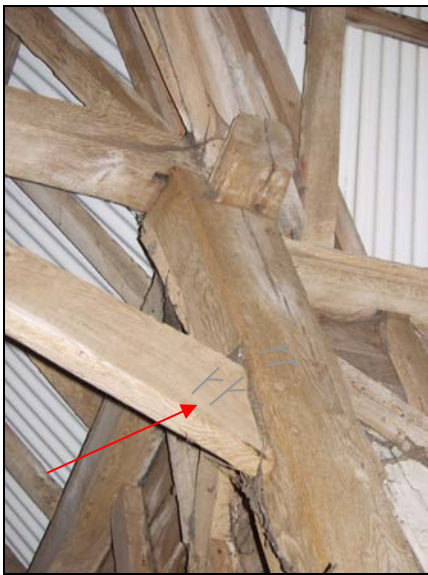
87 Truncated wall-plate at the head of Truss 1, and assembly mark (emphasised and indicated) on brace and post, taken from the south-west
