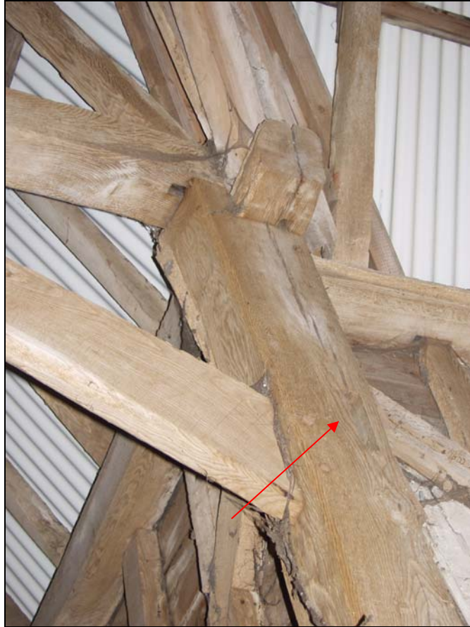
Plate 5 Truncated wall-plate at the head of Truss 1, with mortice (indicated) in the principal post for a former upward brace, taken from the south-west (87)
