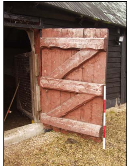
102 Detail of massive ledged and braced door on east side of Building 6 (Unit A), taken from the south-east
