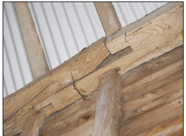
90 Face-halved and bladed scarf joint in west wall-plate of Building 1 (Bay 4), taken from the north-east
