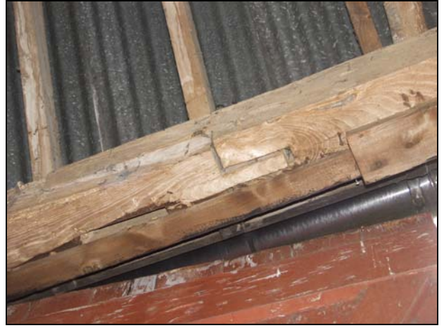
98 Edge-halved and bladed scarf joint in the south wall-plate of Building 2 (Bay 3), taken from the north
