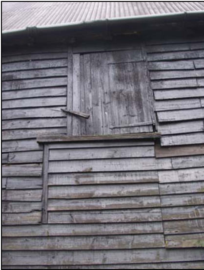
93 Detail of high-set loading door on south elevation of Building 2 (east end), taken from the south
