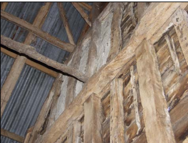
95 Detail of redundant soffit groove in the east wall-plate (Building 2), taken from the south-west
