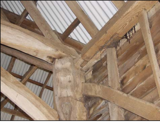
91 Detail at head of west side of Truss 2 (Building 1) and face-halved and bladed scarf joint in wall-plate (Bay 3), taken from the south-west
