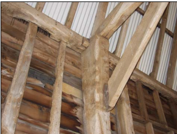
89 Head of west side of Truss 2 (Building 1) with face-halved and bladed scarf joint in the wall-plate, taken from the south-east
