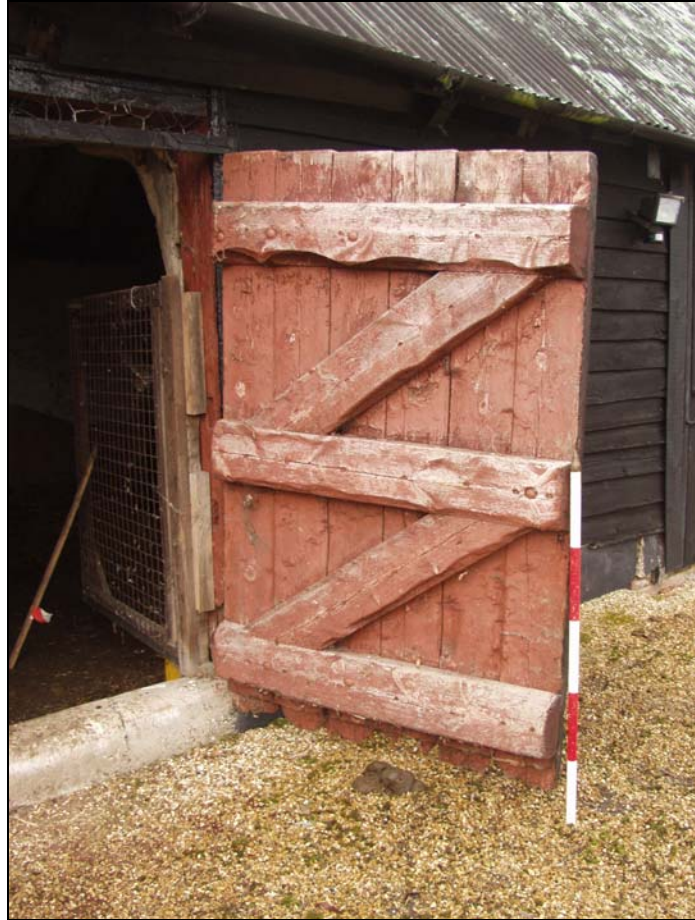
Plate 13 Detail of robust ledged and braced door on east side of Building 6 (Unit A), taken from the south-east (102)
