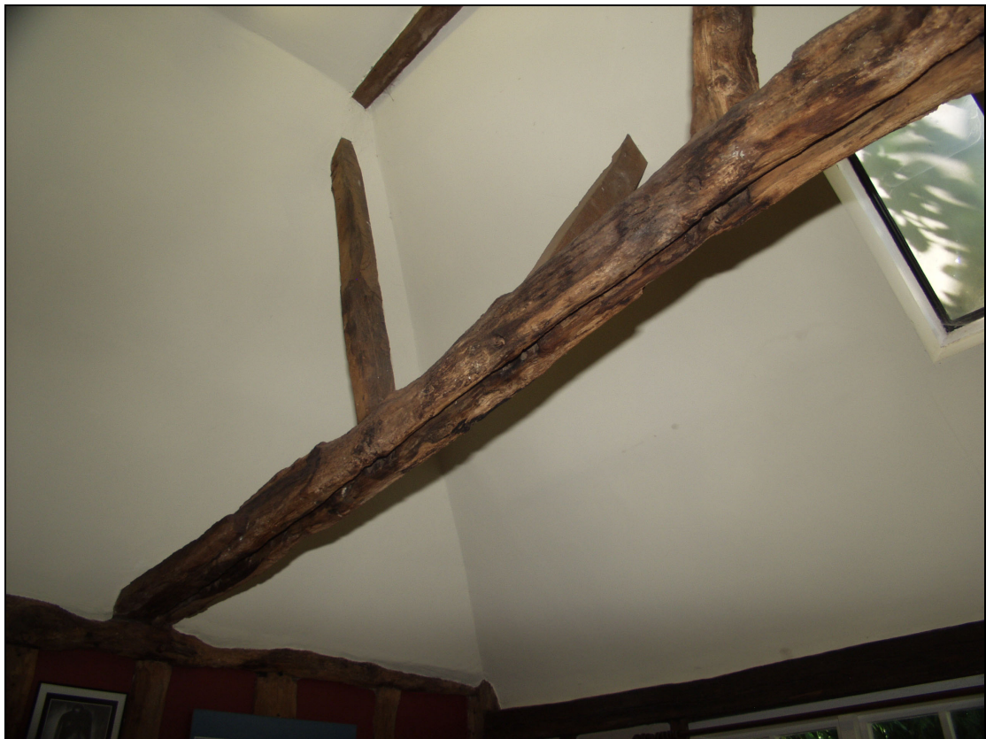
Plate 8 Detail of tie-beam in Room 1 showing groove and redundant mortices, taken from the north-east (53)
