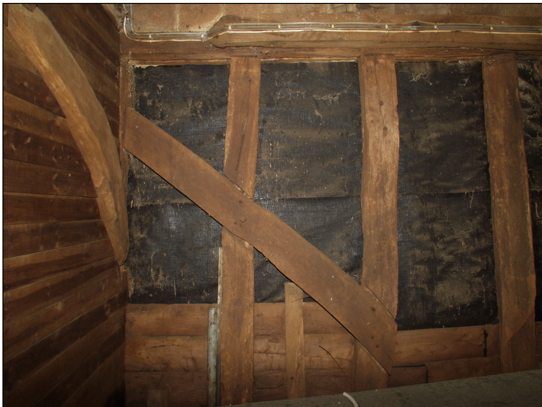
Plate 6 Detail of original 16th century brace on north wall of the barn (Bay 4), taken from the south (72)
