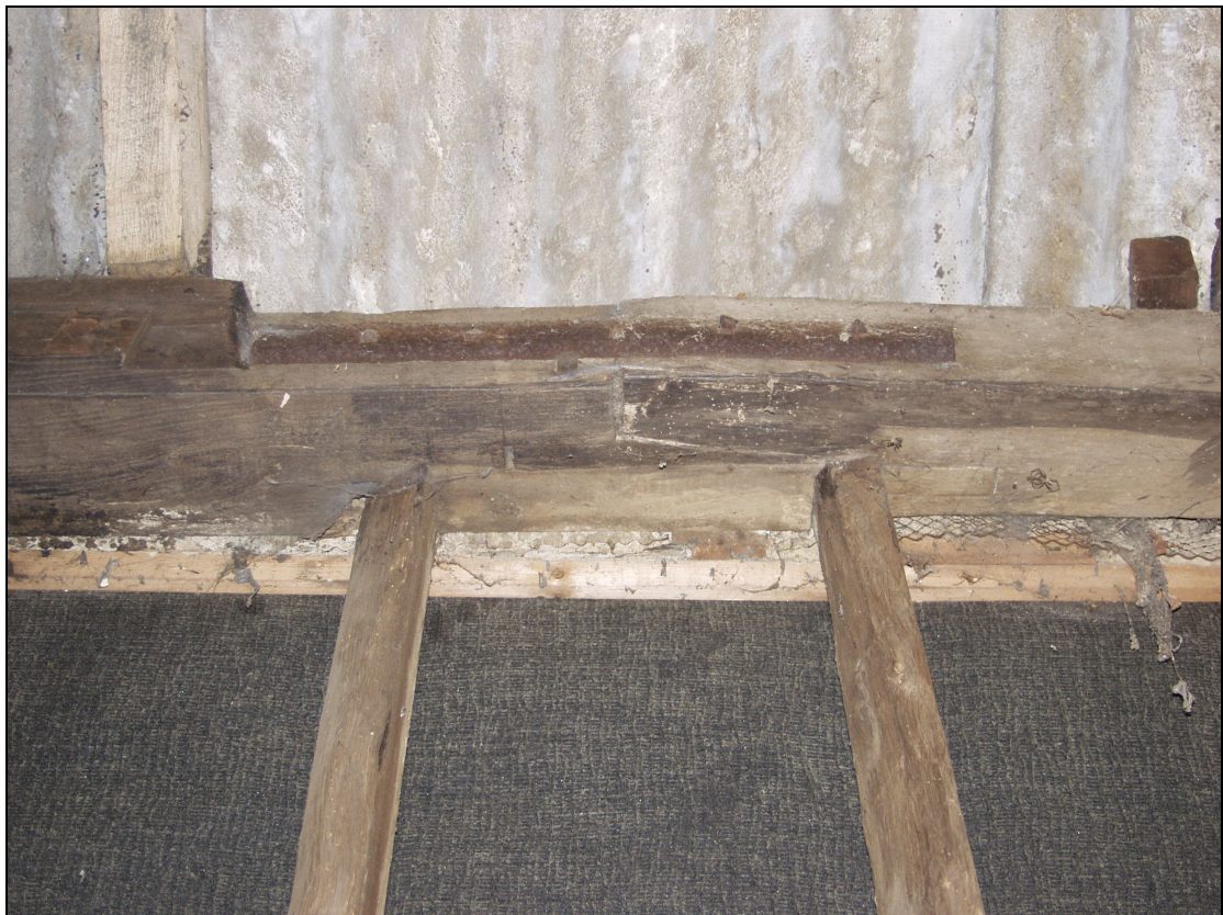
Plate 4 Scarf joint in the south wall-plate of the barn (Bay 2), taken from the north (35)
