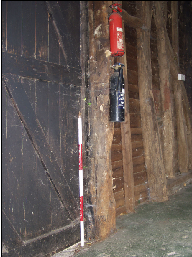
Plate 5 East door jamb of barn entrance showing mortises for locking bars and a threshing leap, taken from the south-west (32)
