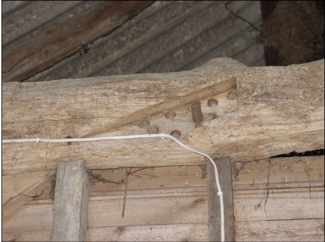
Plate 7 Redundant mortice on the west face of Truss 5, taken from the west (42)
