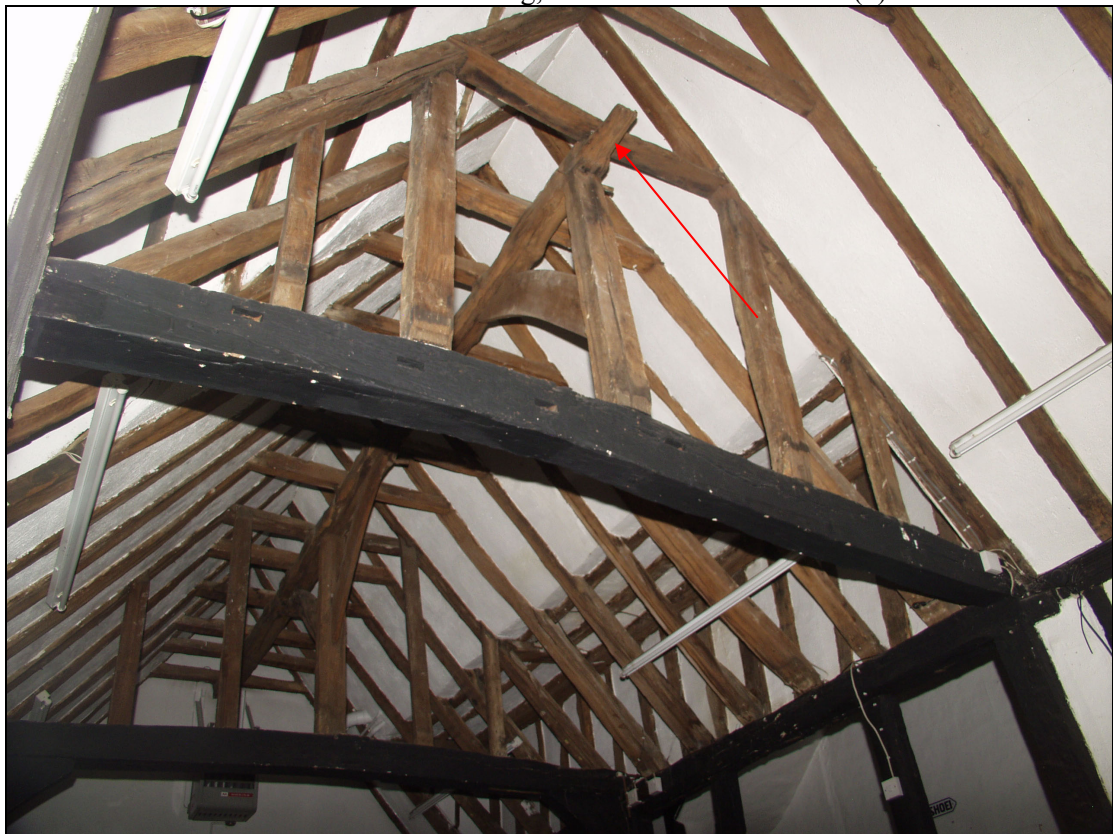
Plate 2 Roof structure of the central range showing crown-purlin stump (indicated) to the original gable end, taken from the south-east (40)
