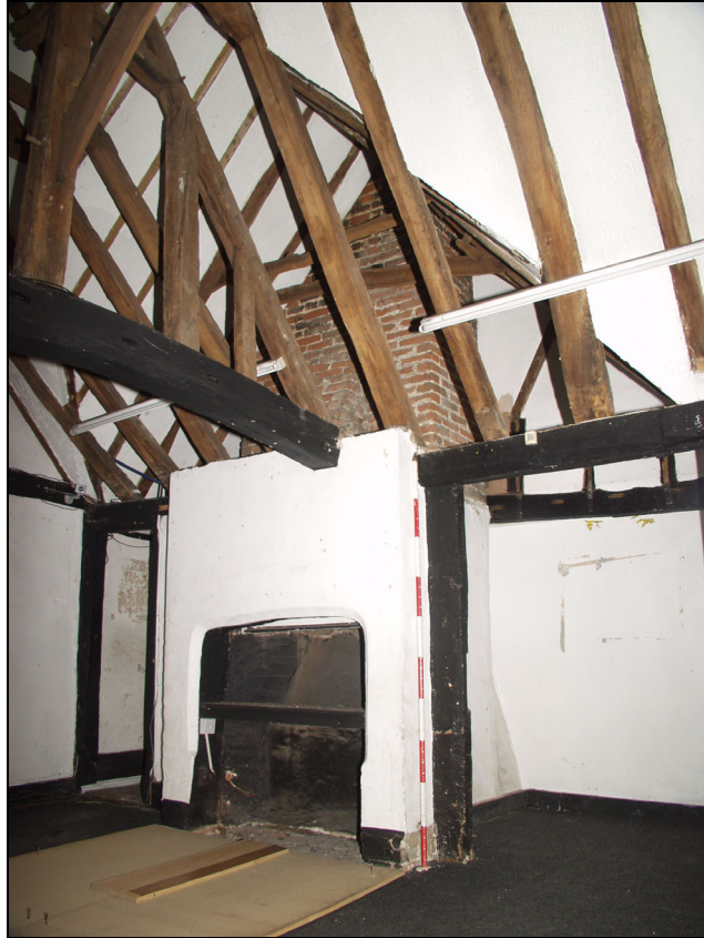
Plate 3 Detail of fireplace and chimney extension in Room 7, first floor of the central range, taken from the north-west (42)
