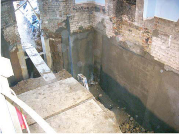
DP 7. N and E walls of the house inside the basement. Taken from SW.
