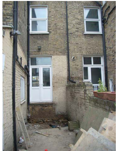
DP 4. Rear of the house with excavation for light well. Taken from SSE.
