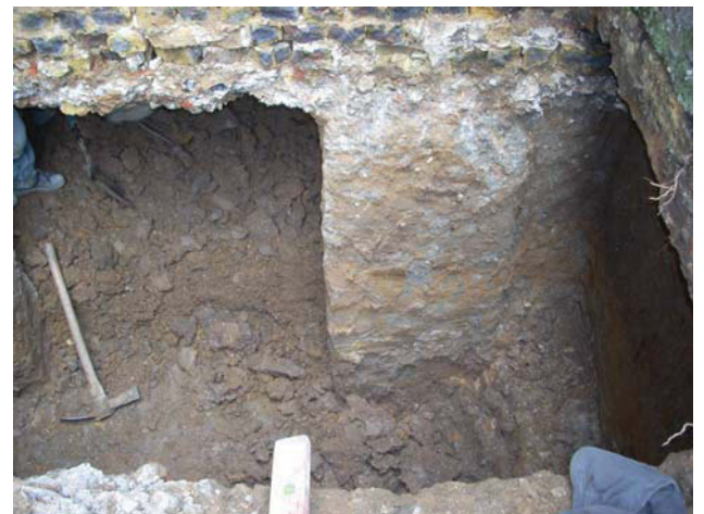
DP 12. Excavation for the light well to the rear of the house. Taken from SSE.
