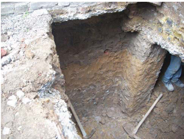
DP 11. Excavation for the light well to the rear of the house. Taken from SE.
