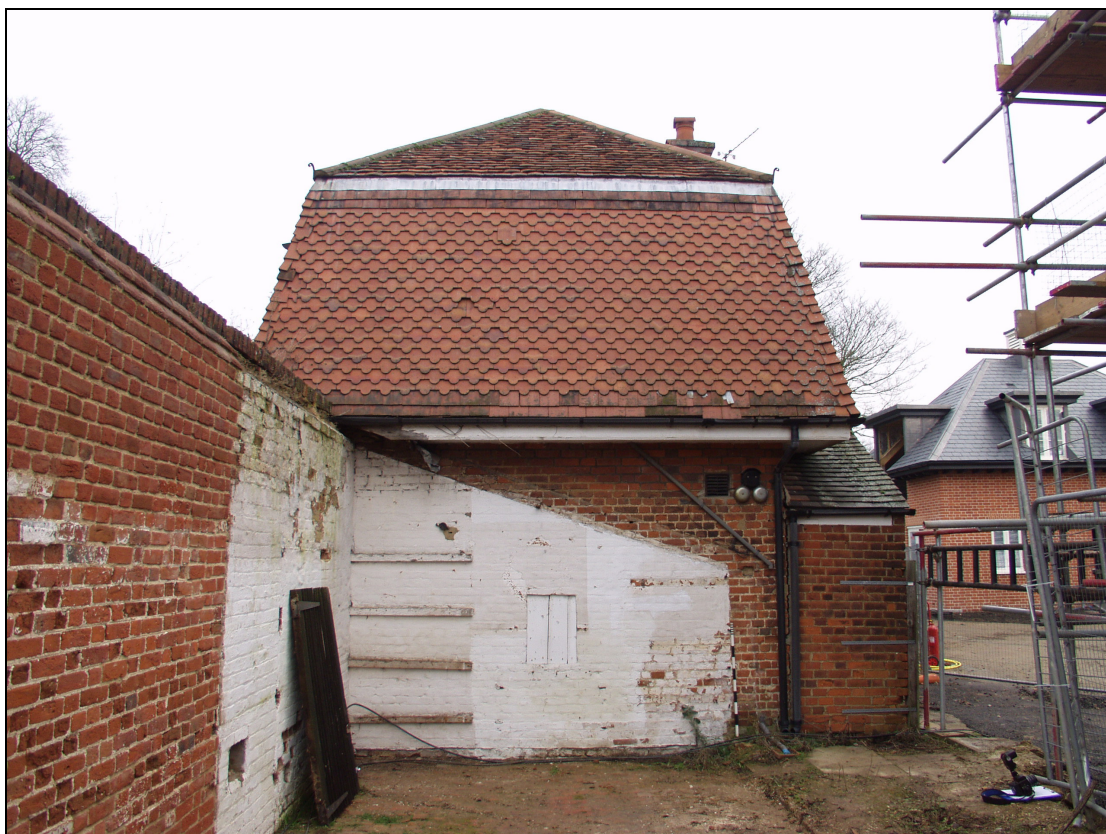
1 South elevation of Lime Cottage, forming the side wall of the demolished outbuilding, taken from the south (2)
