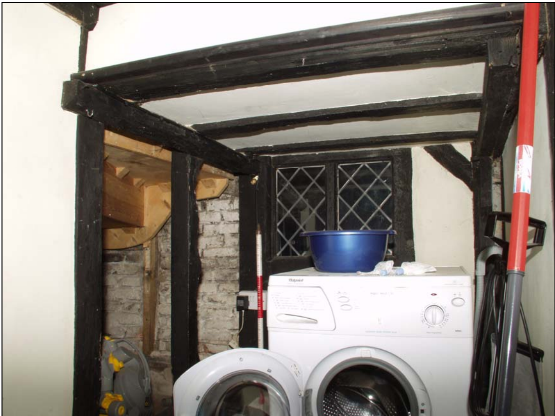
14 Modern stair structure on ground floor of stair-turret, taken from the south (21)
