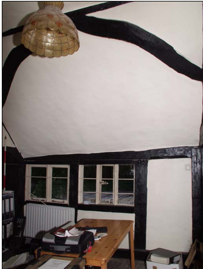
11 Bedroom to west side of chimney stack in 16 th century east – west range, taken from the south-east (37)
