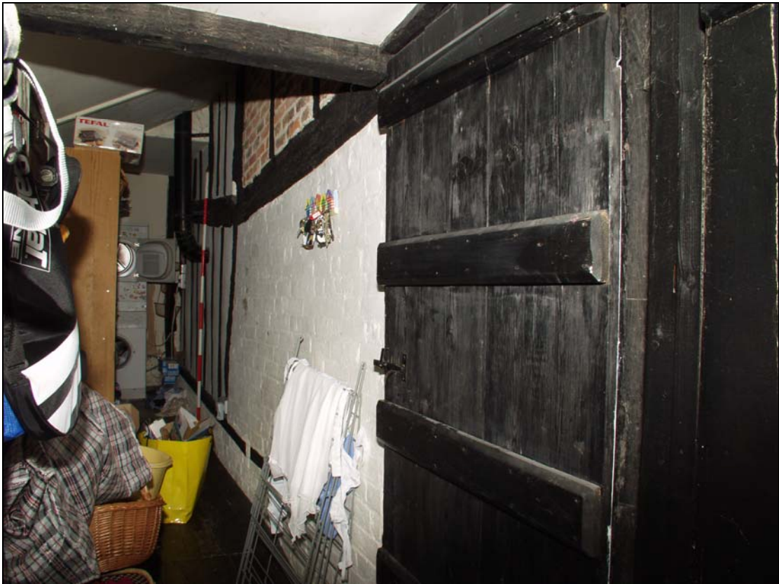
20 North wall of 16 th century east – west range now enclosed by outshuts, taken from the west (19)
