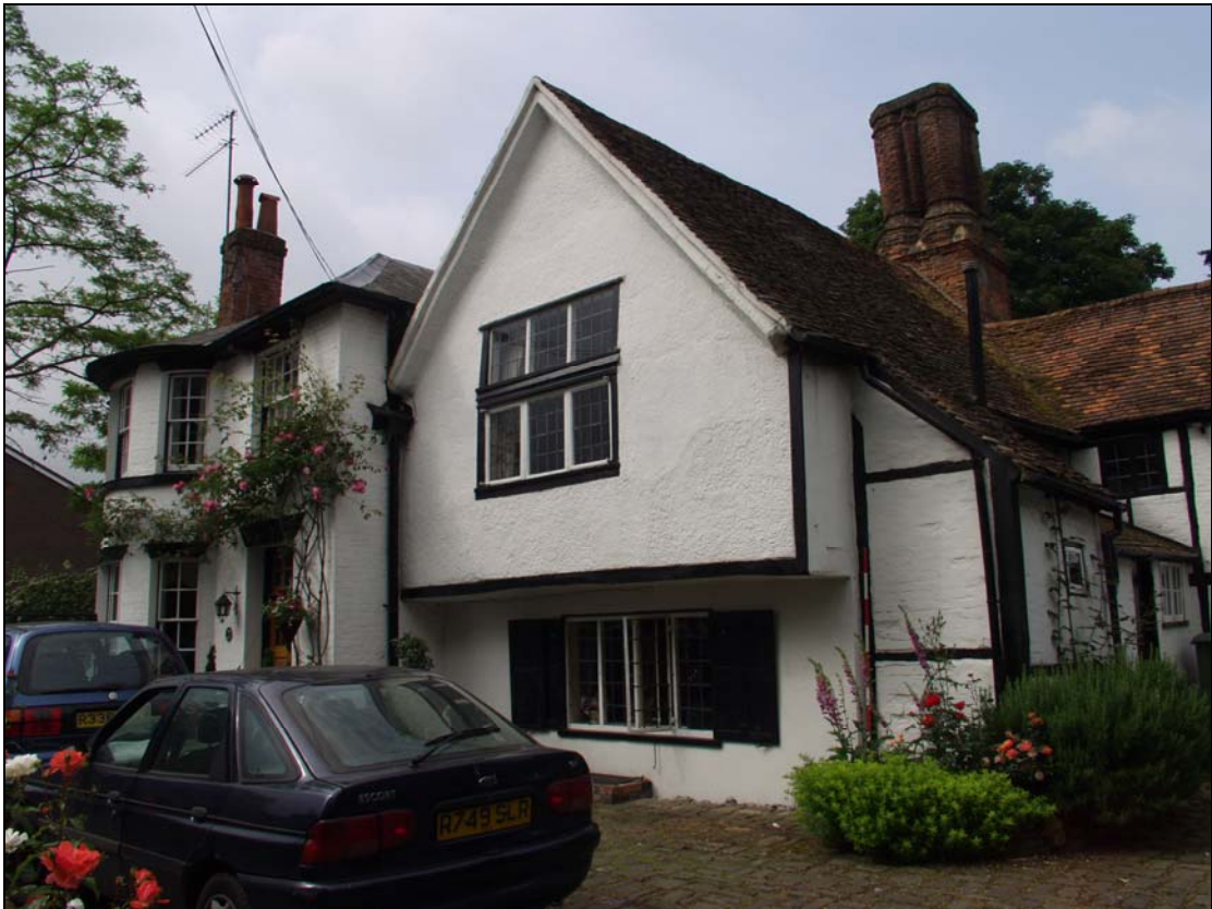
2 East elevation of 16 th century jettied range, outshuts (right) and 1830s wing (left), taken from the north-east (5)
