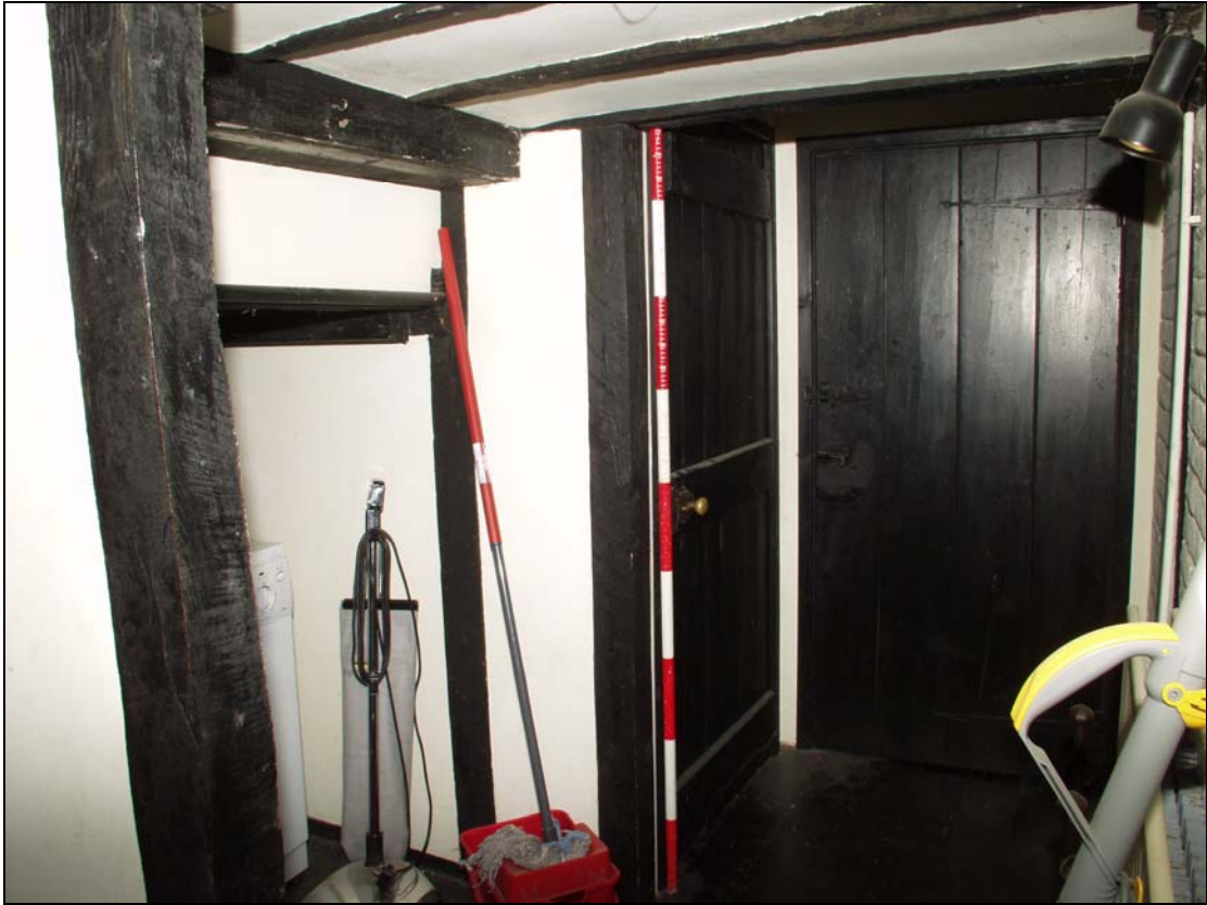
15 Modern doors and bathroom partition on ground floor of stair-turret, taken from the south-west (20)
