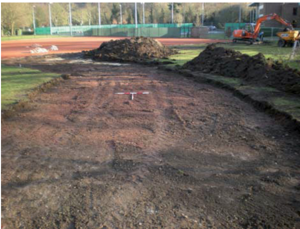
DP3 Area of access road and north part of a new tennis court after ground reduction.
