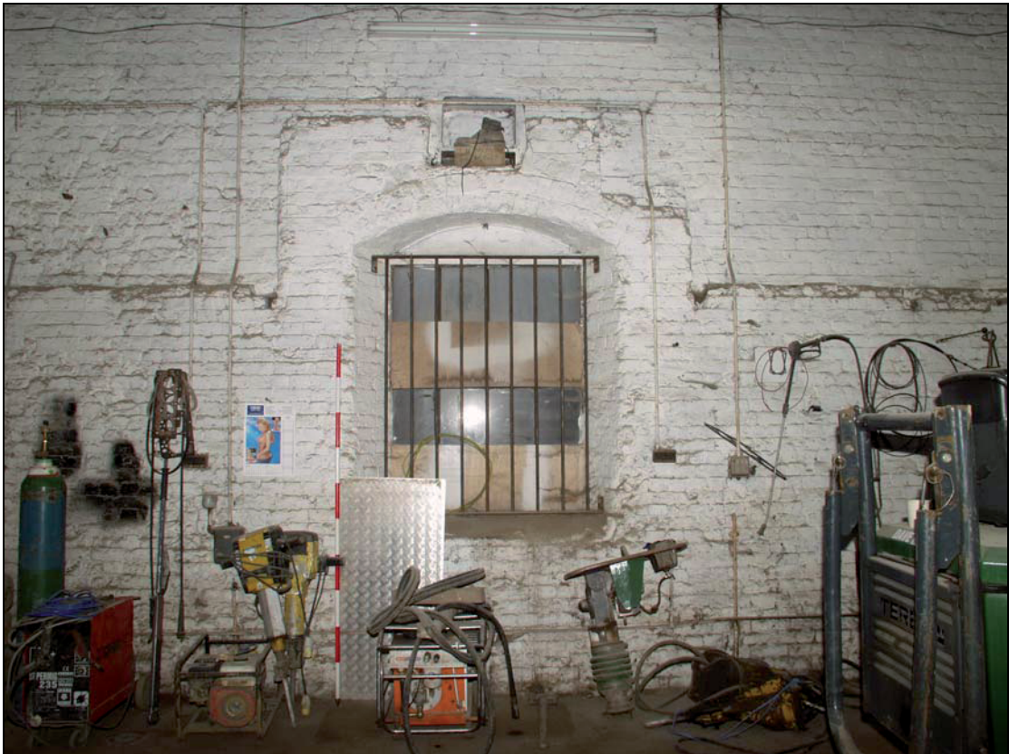
4 Robust brickwork surrounding window in Building 1 – east bay, taken from the west (22)
