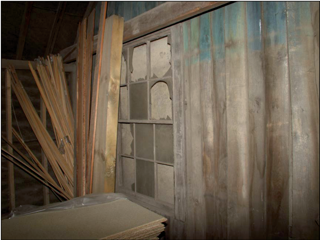
18 19 th century window in north wall of Building 4 – south section, taken from the north-west (36)
