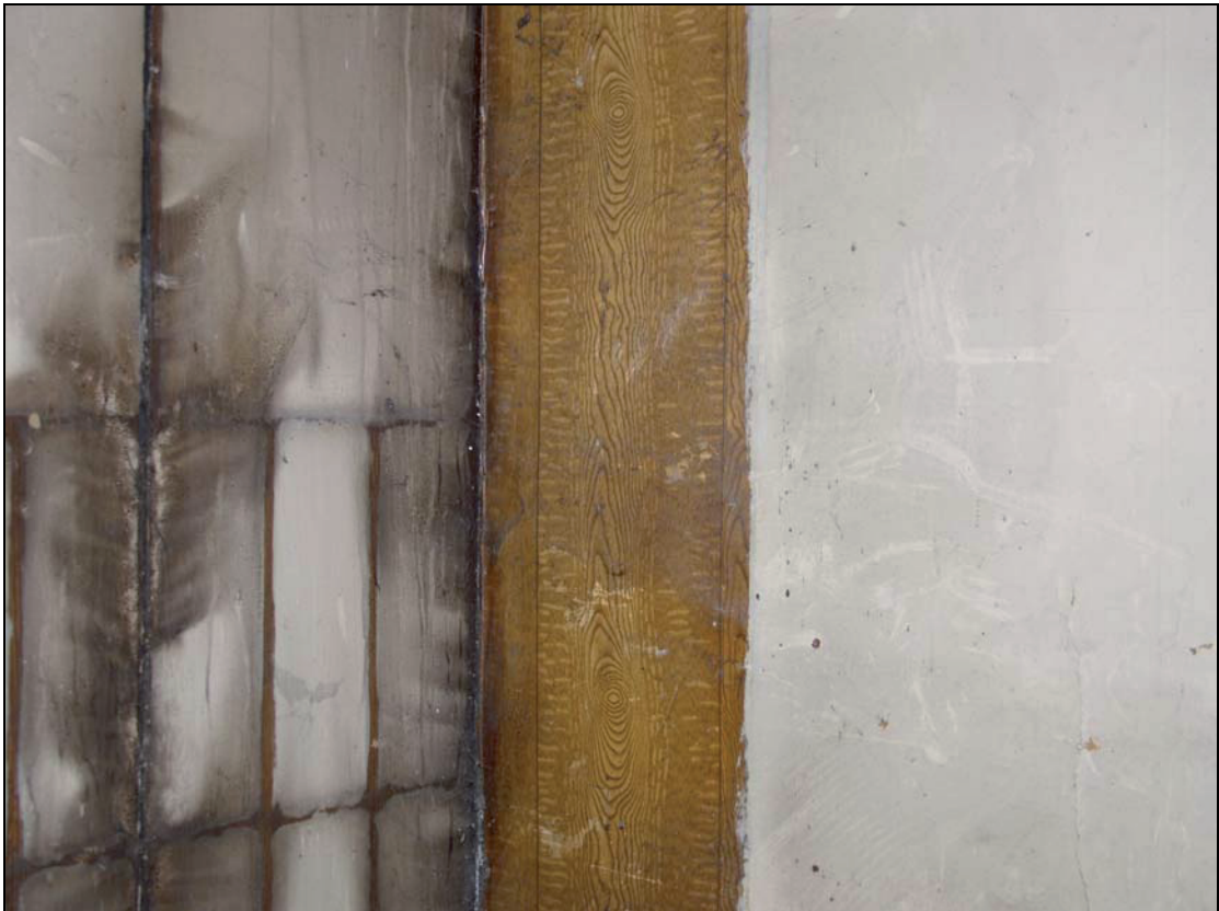
14 Grained match-line boarding on west wall of office in Building 3, taken from the east (33)
