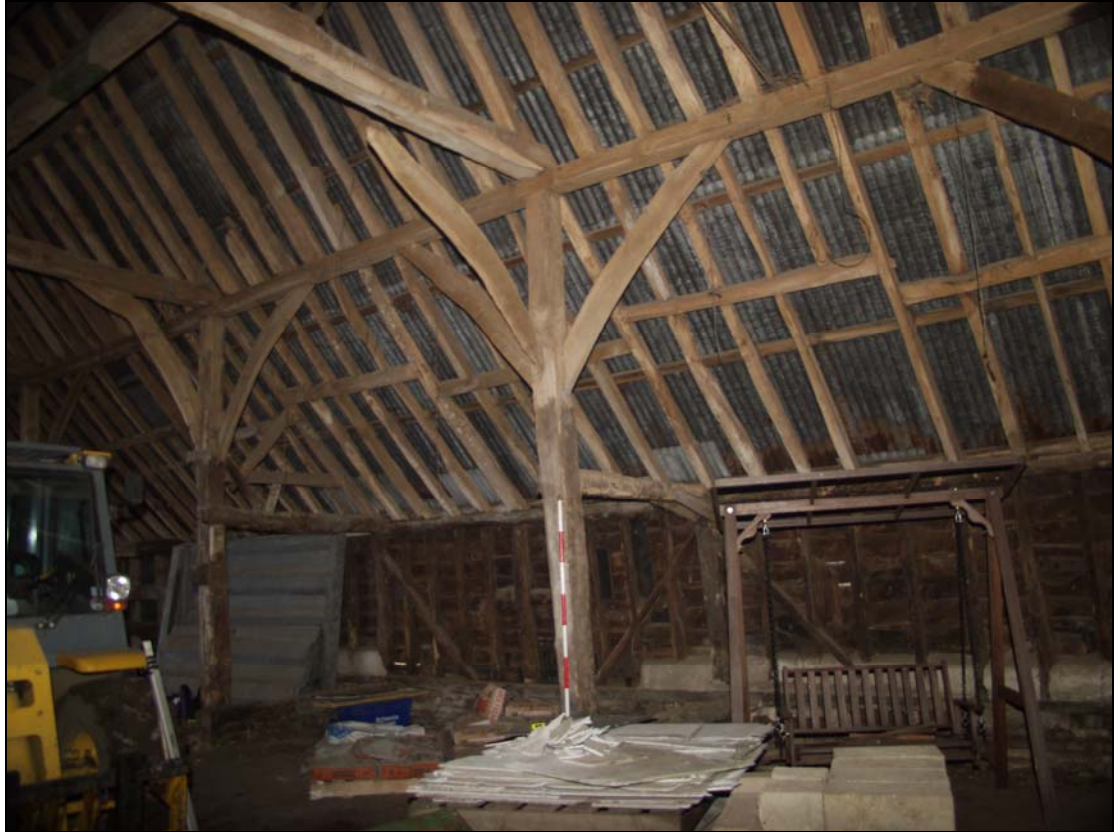
Plate 3 West side of Bays 1 and 2 (Building 1) showing truss configuration, taken from the north-east (51)
