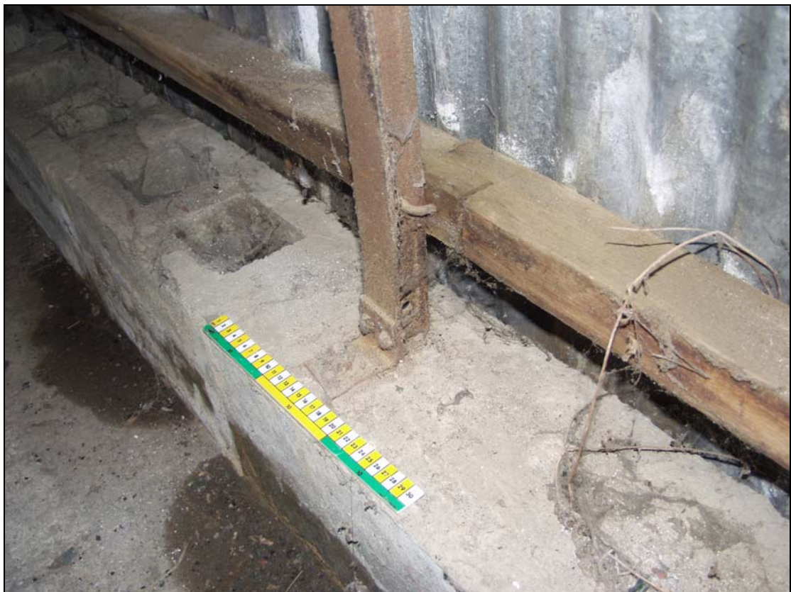
Plate 8 Construction detail of Building 2 at base of a truss, taken from the west (29)
