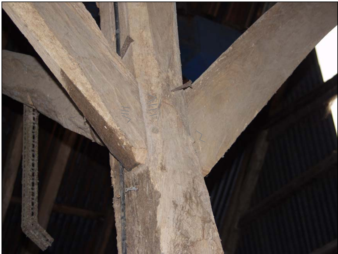
Plate 6 Assembly marks (emphasised) on west side of Truss 4, (Building 1), taken from the north-west (56)
