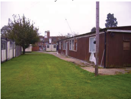
DP23 Range of modern chalet and pre-fab structures located to the rear of the main Bush Hall Hotel building, view south-eastwards
