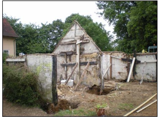
2 Outbuildings under renovation. Sample Section 1 is located within the nearest trench. Looking south.
