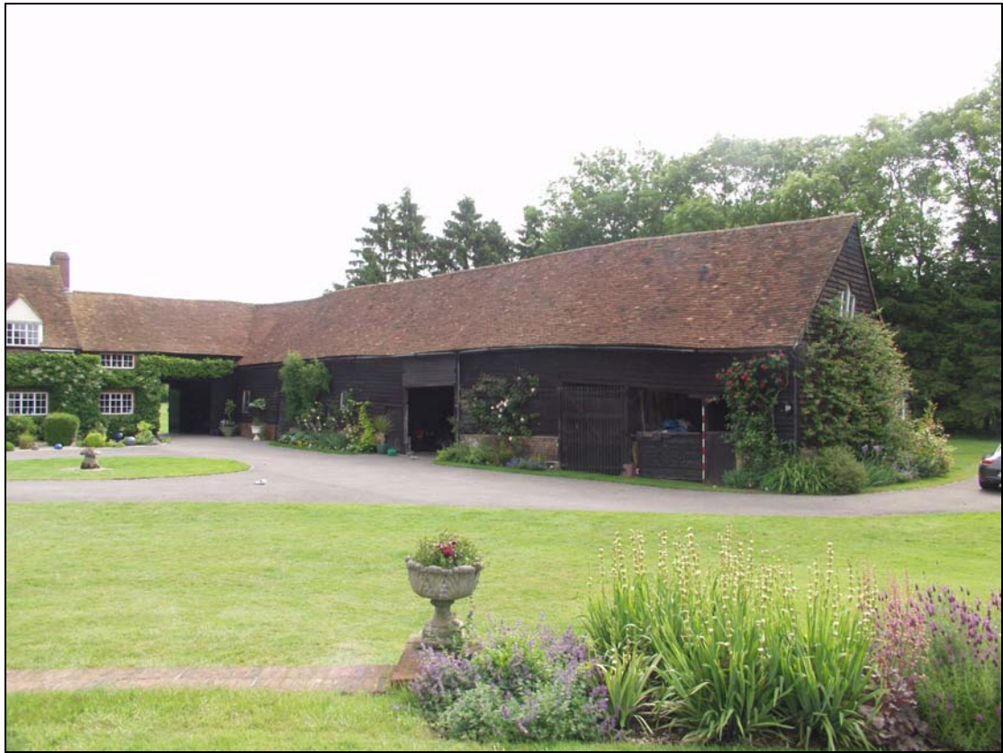
Plate 3 West elevation of the assessment range with the carriageway to the rear, taken from the south-west (08)
