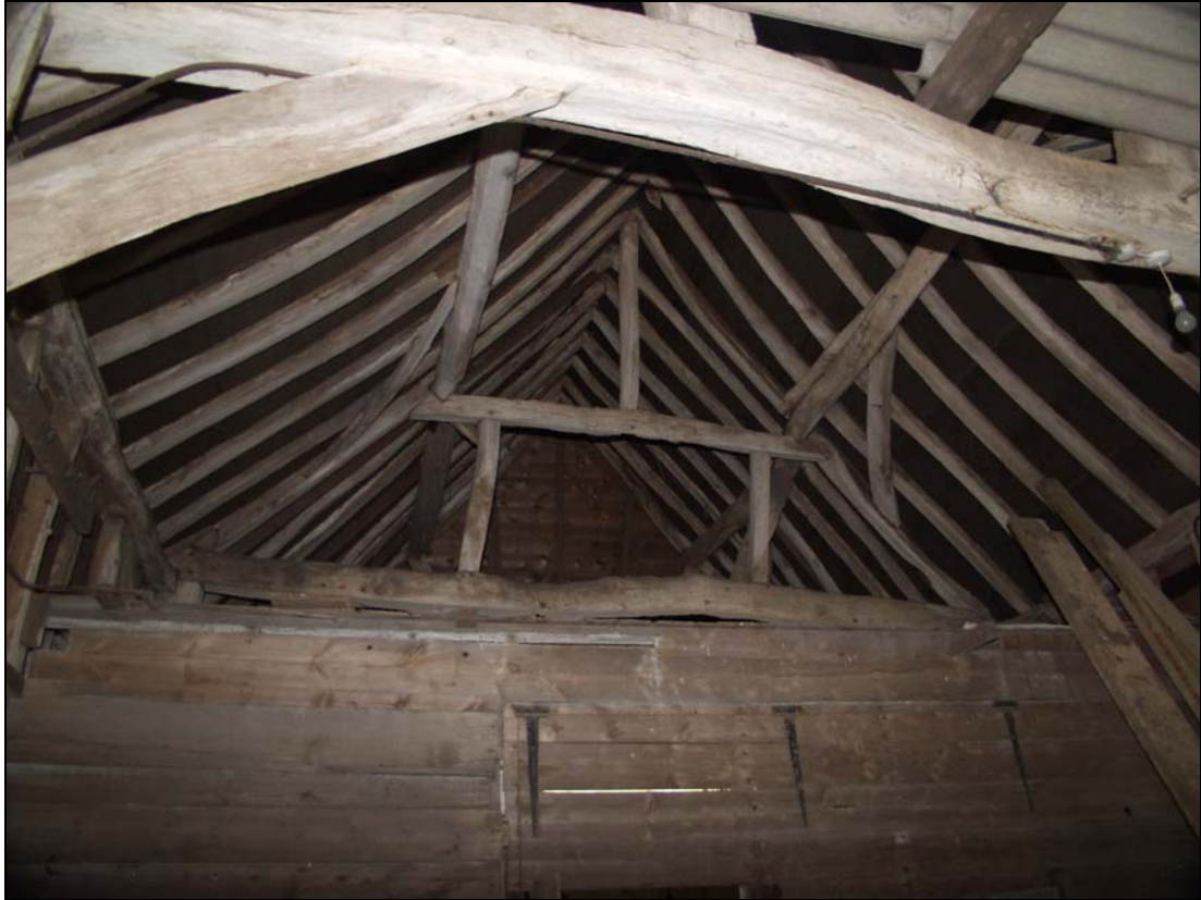
Plate 5 View of roof structure over Unit 3, north outer truss of the 15th century barn, taken from the south-west (21)
