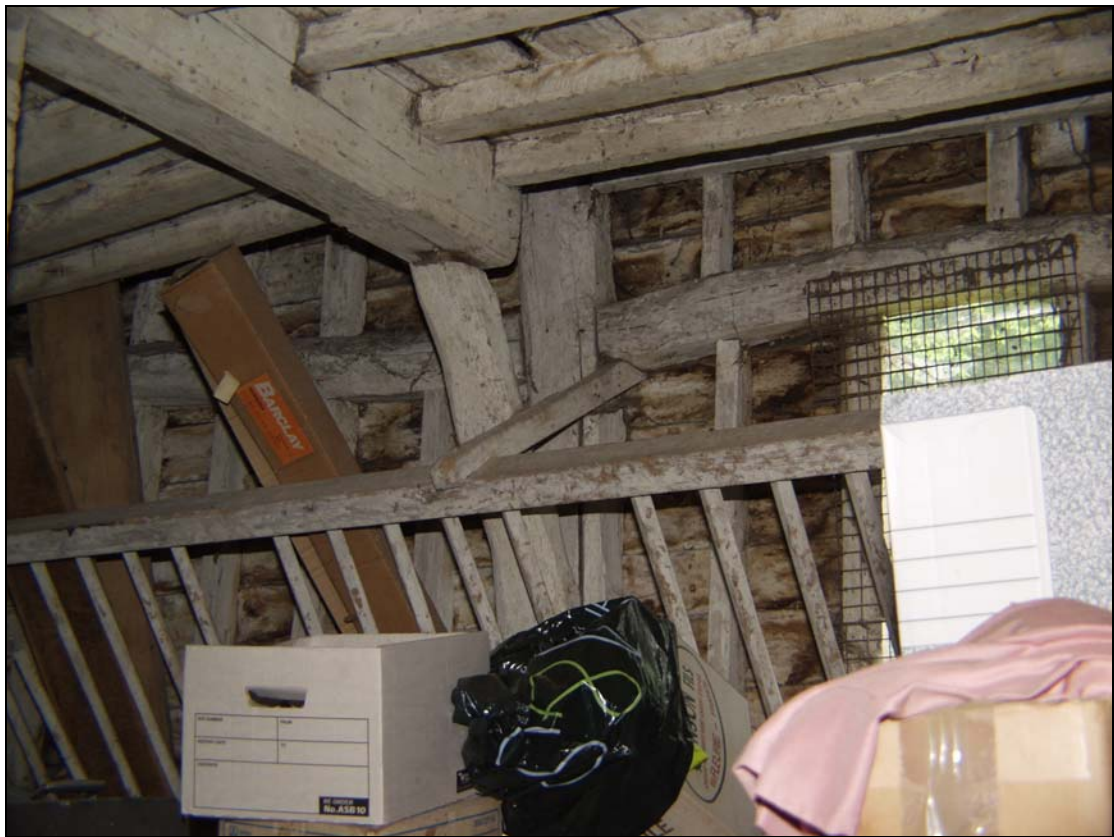
Plate 4 Detail of the east wall of Unit 1 showing floor joist and crude brace, taken from the west (15)
