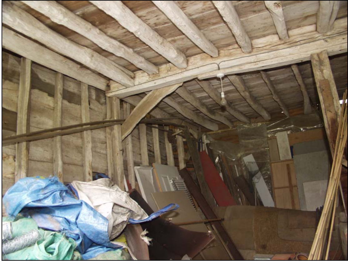
Plate 9 Ground floor of the central bay of Unit 5, taken from the west (29)
