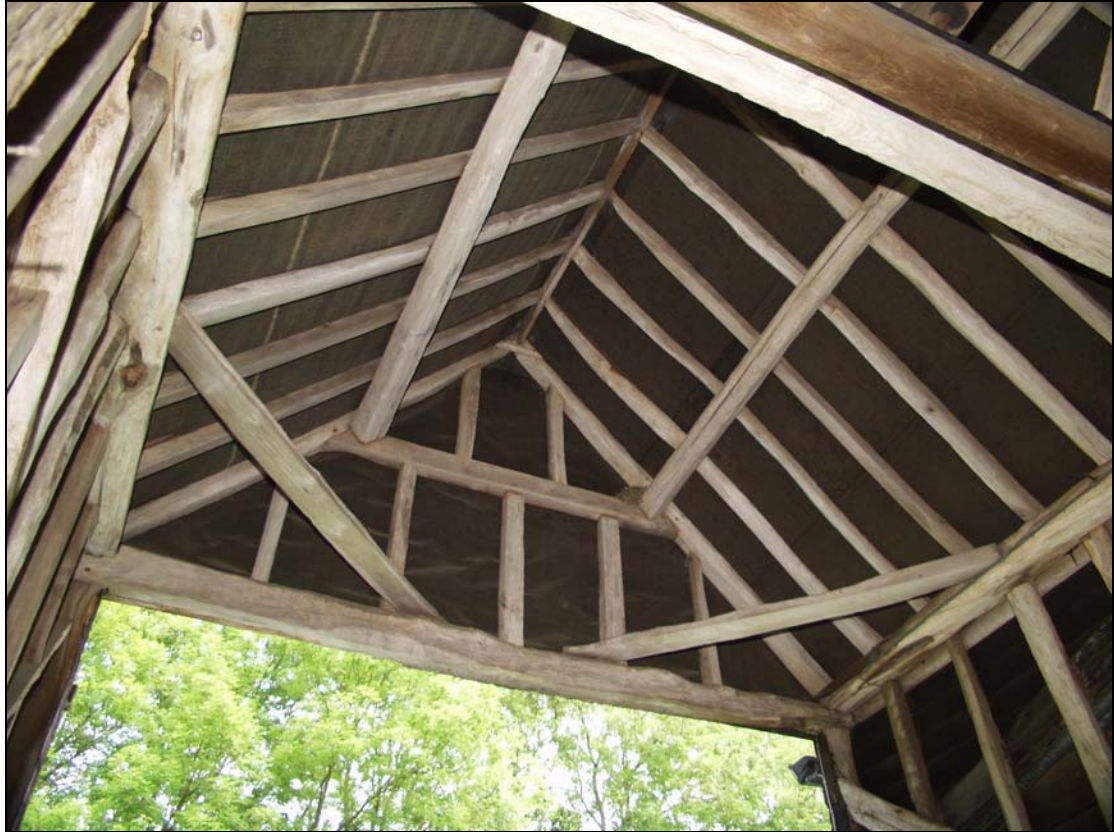
Plate 7 Roof form of the porch on the east side of Unit 4, taken from the north-west (25)
