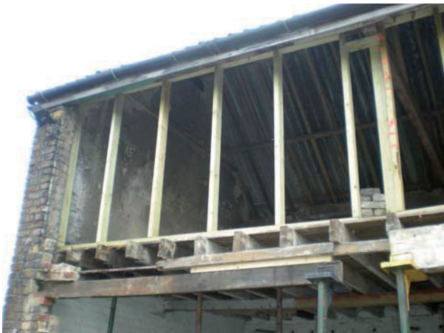
DP 29. Floor joists in former stable, Building A, first floor. Taken from S.
