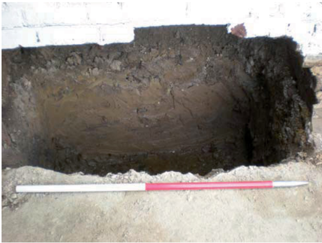
DP 33. Former stable, Building A, NE corner. Foundation pit/trench. Taken from N.
