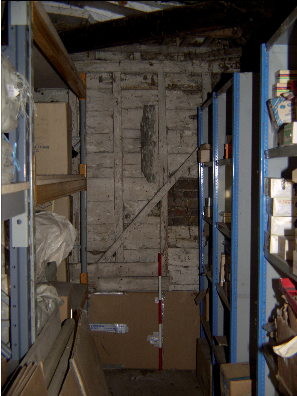
6 Detail of southern section of timber framed wall to east end of single storey section of Building A (17)
