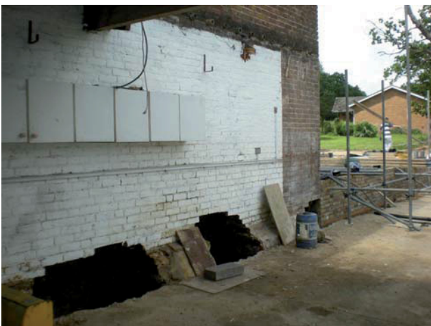
DP 35. N wall of Building A with foundation pits/trenches. Taken from NE.
