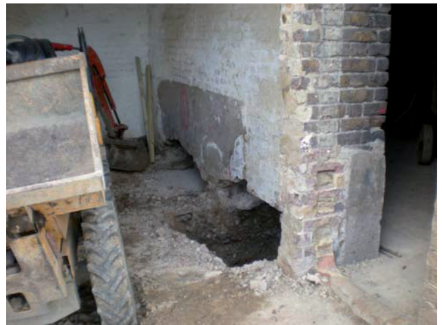
DP 30. E wall of former stable, Building A, showing foundation pit/trench. Taken from SW.
