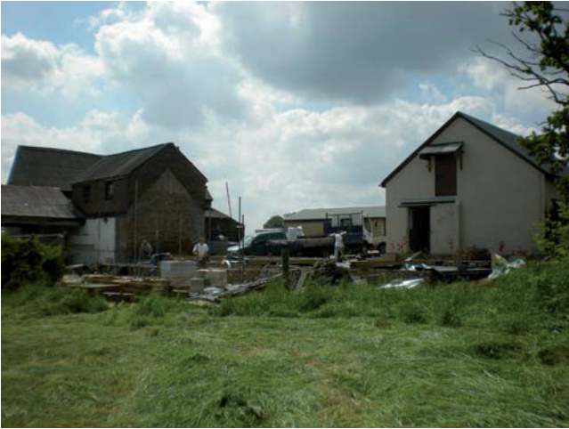
DP 25. General view of the site, showing the former stable (Building A) to the left and Building B to the right. Taken from NNW.
