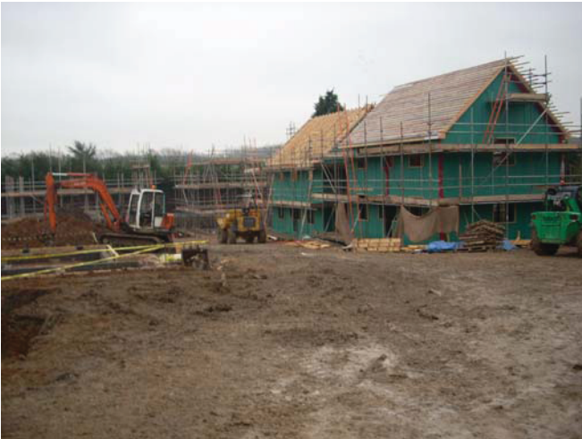
DP 3. General view of the site, plot G on foreground. Looking from NW. January 2009.
