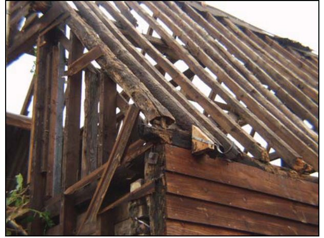
42 Detail of the south-west corner of Building 3 after removal of the roof covering, taken from the south-west
