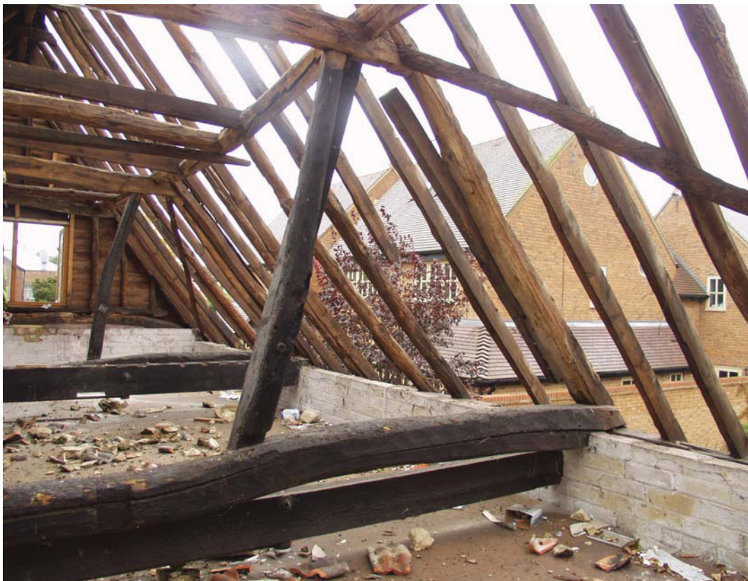
Plate 8 South side of Building 3 at upper level, after removal of the roof covering, taken from the north-west (DP 41)
