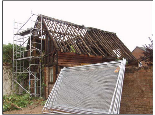
32 View of Building 3 after removal of the roof covering, taken from south-west
