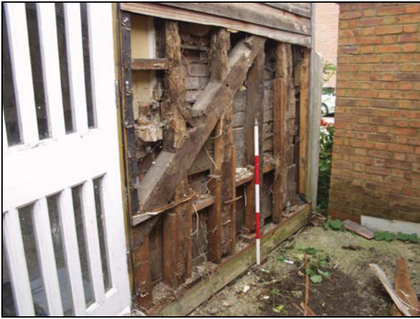
31 Timber-framing of the east bay, south side of Building 3, taken from the south-west
