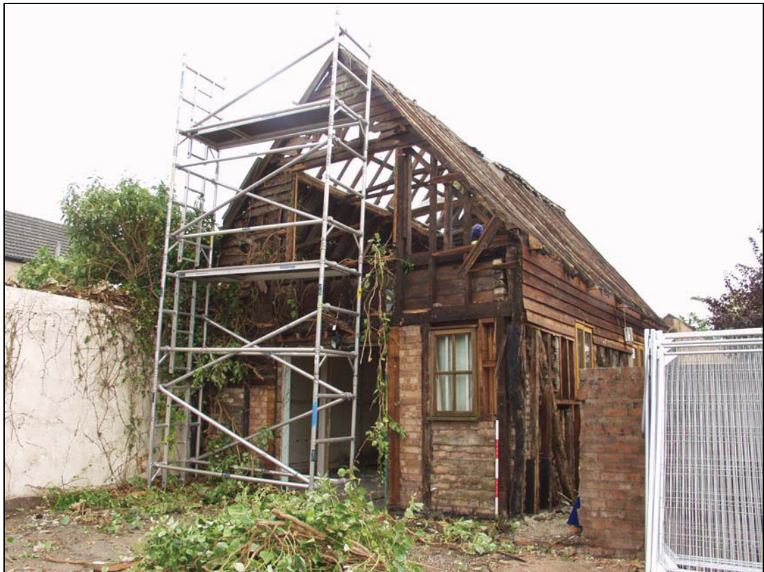
Plate 6 View of Building 3 after removal of the roof covering and external weatherboarding, taken from south-west (DP 33)
