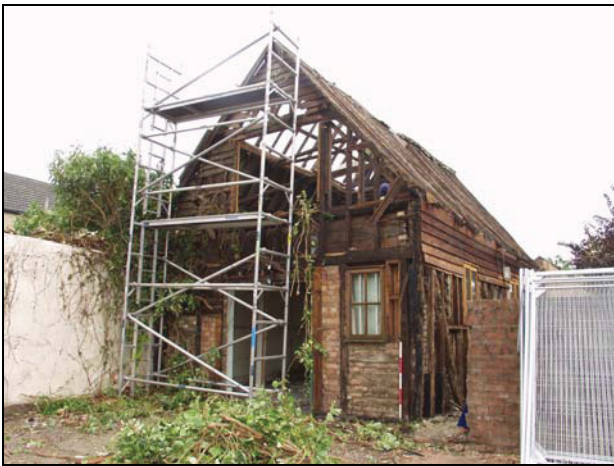
33 View of Building 3 after removal of the roof covering and external weatherboarding, taken from south-west
