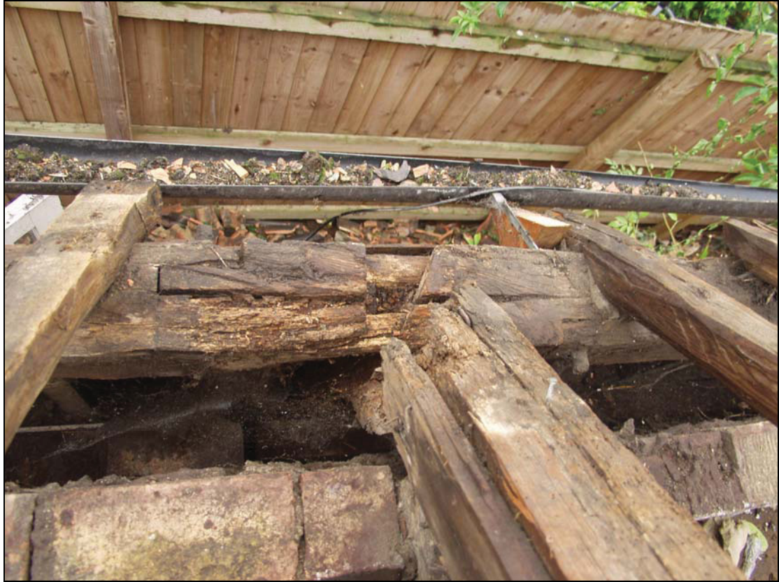
Plate 9 Detail of scarf joint in the south wall-plate of Building 3, taken from the north (DP 36)
