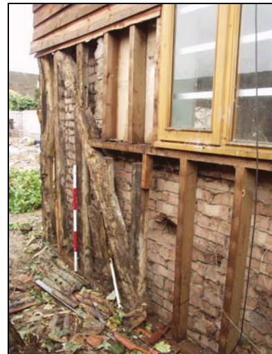
34 Timber-framing of the west bay, south side of Building 3, taken from the south-east
