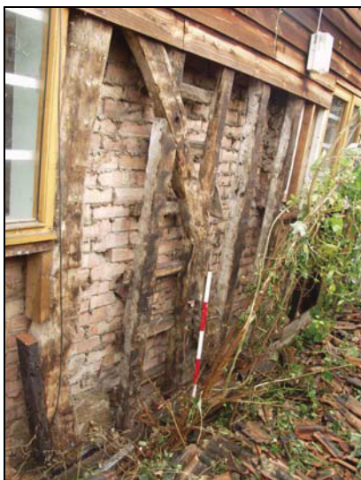
35 Timber-framing of the central bay, south side of Building 3, taken from the south-west
