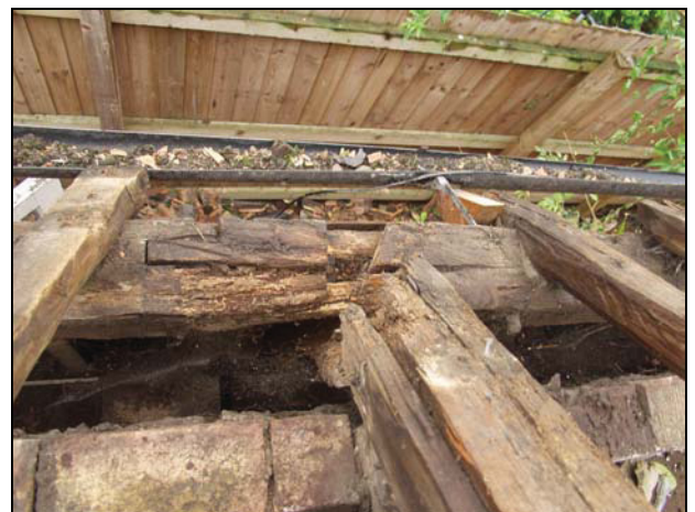
36 Detail of scarf joint in the south wall-plate of Building 3, taken from the north
