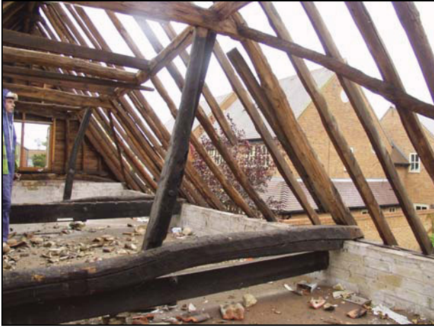
41 South side of Building 3 at upper level, after removal of the roof covering, taken from the north-west
