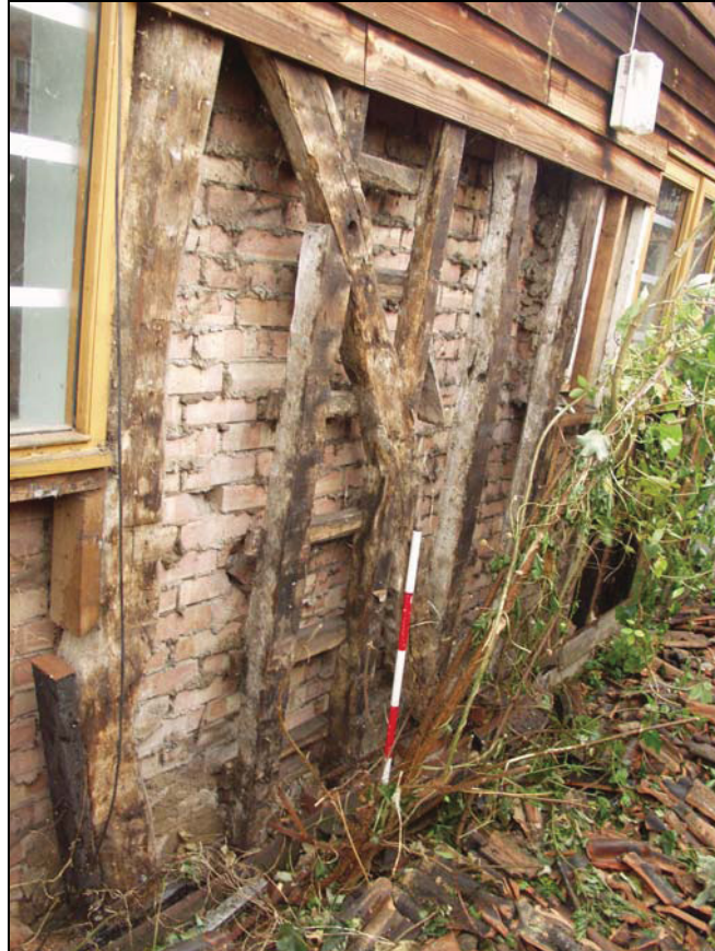
Plate 7 Timber-framing of the central bay, south side of Building 3, taken from the south-west (DP 35)
