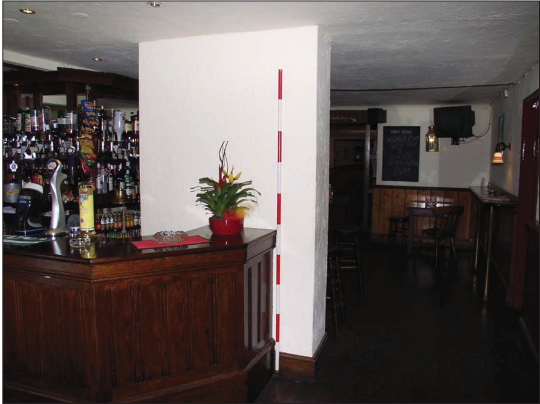
3 Free-standing 18 th century chimney stack between Rooms 2 and 3, principal range. Taken from the south (8)
