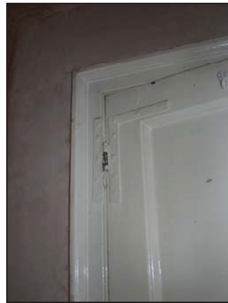
72 Original hinge on 18 th century door to Room 9, first floor, taken from the west
