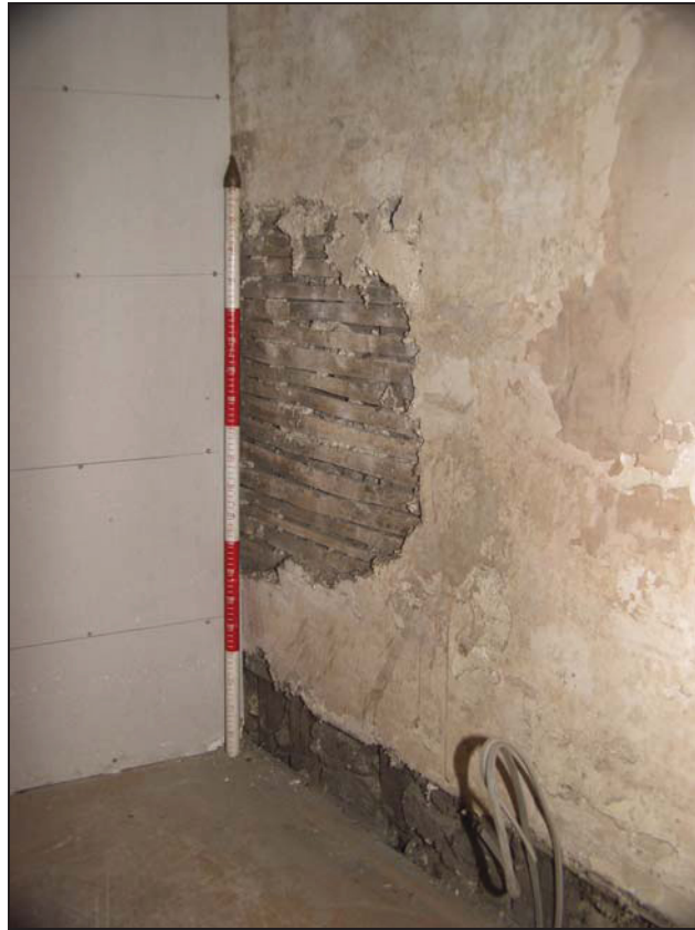
23 South wall of Room 10 (first floor of principal range) showing exposed lath and plaster, taken from the north-west (42)
