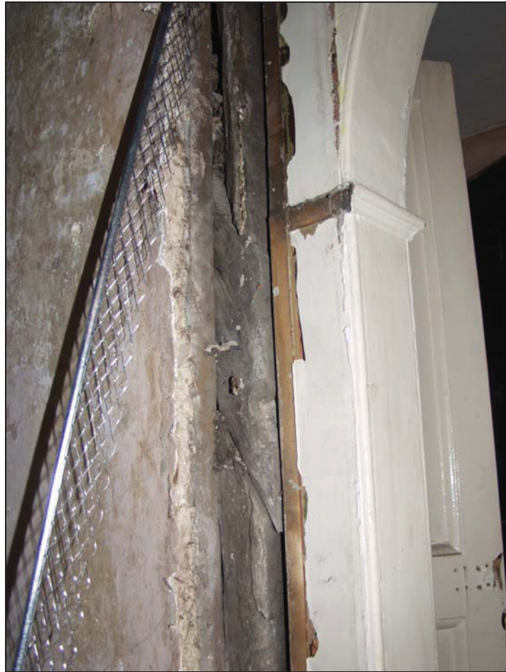
25 Detail on south side of entrance to Rooms 10 and 11 showing possible truncated primary brace, taken from the north-east (73)
