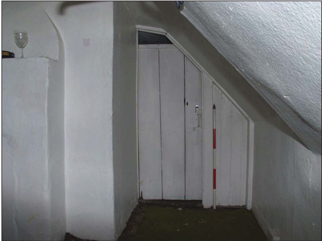
27 Boarded door (possibly of 18 th century date) to Room 14, principal range, taken from the south (25)
