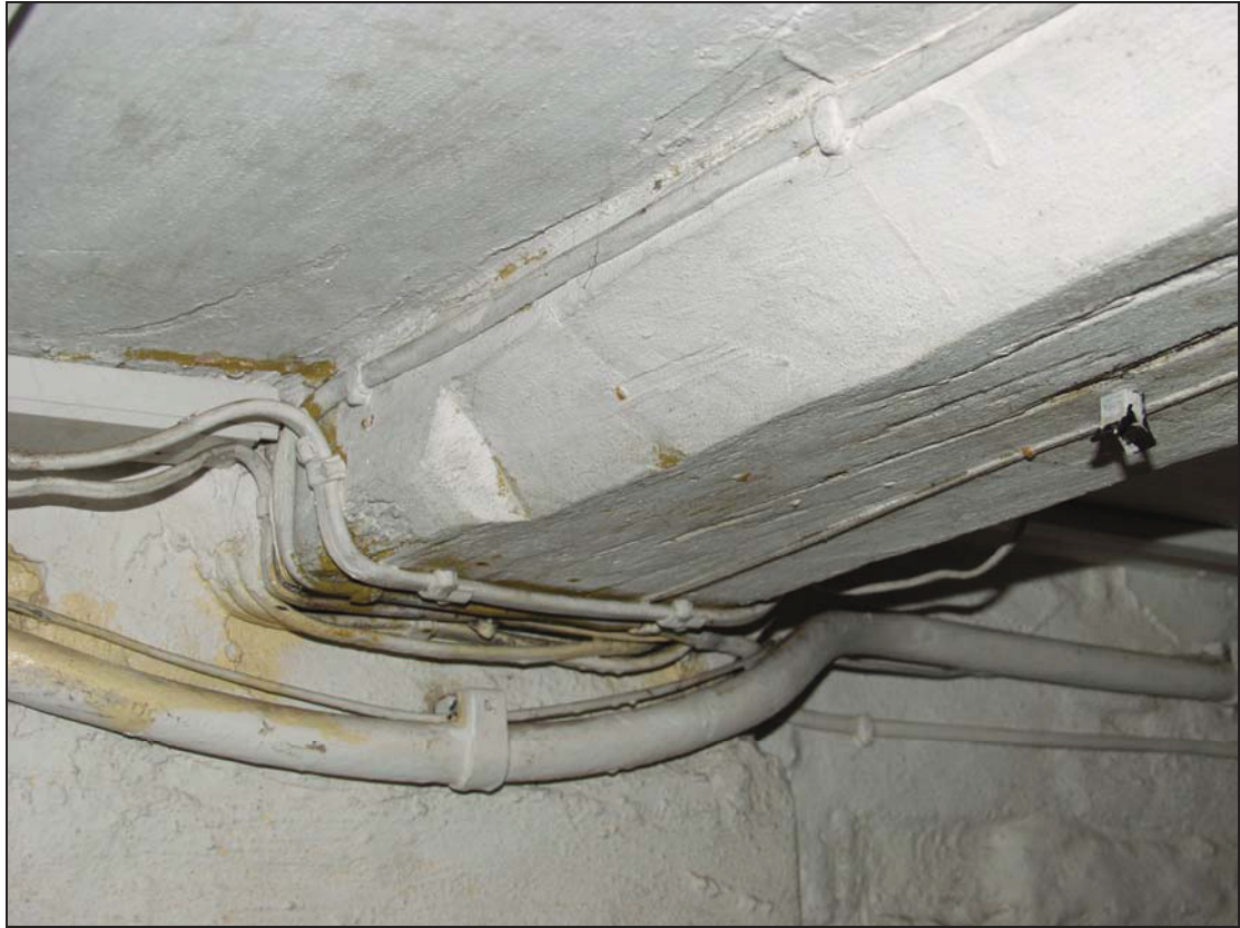
17 Elongated lamb's tongue chamfer stop on ceiling joist above Room 8, cellar, taken from the south-east (13)
