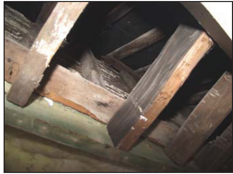
50 View of rear side of lath and plaster covered studwork forming the walls to the attic
