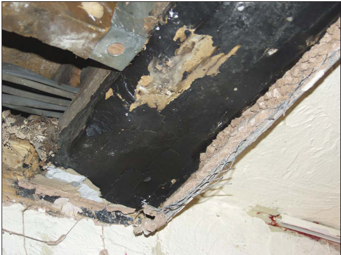
8 Binding joist in Room 3 showing chamfers and run-out stops, taken from the south-east (38)
