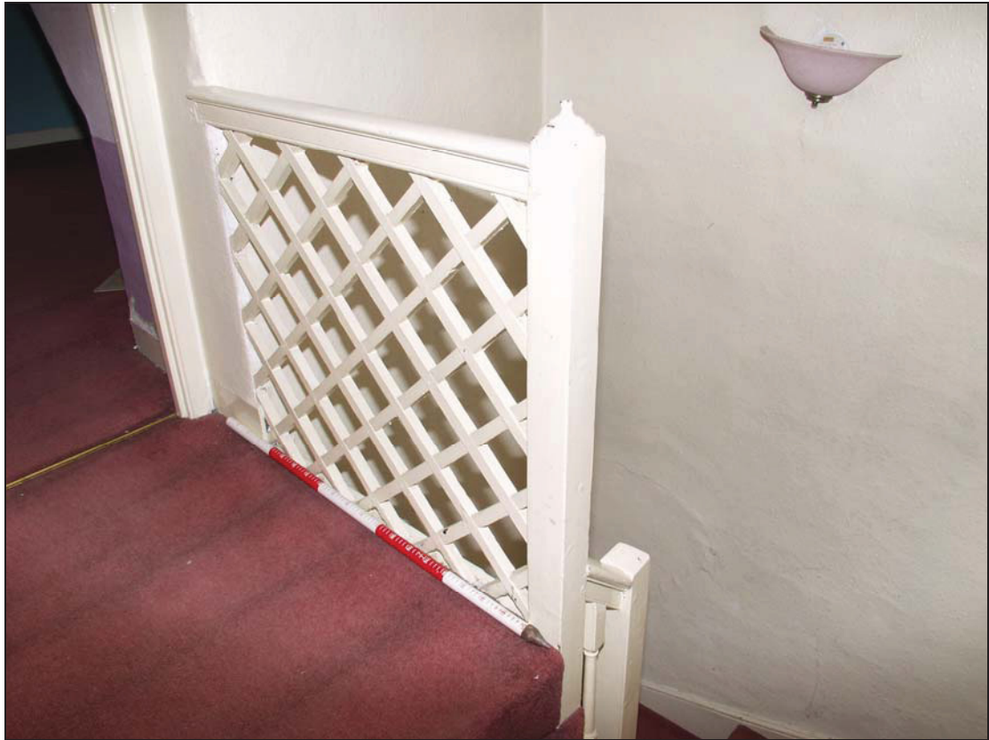
15 Lattice screen in place of balusters on attic landing, principal range, taken from the north-east (22)
