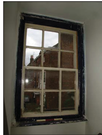
58 Sash window on the east wall of the rear range, first floor, taken from the west
