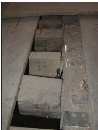
53 Exposed floor joists in Room 11 showing assembly markings, taken from the east
