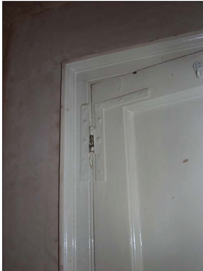
20 Original hinge on 18th century door to Room 9, first floor of principal range, taken from the west (72)
