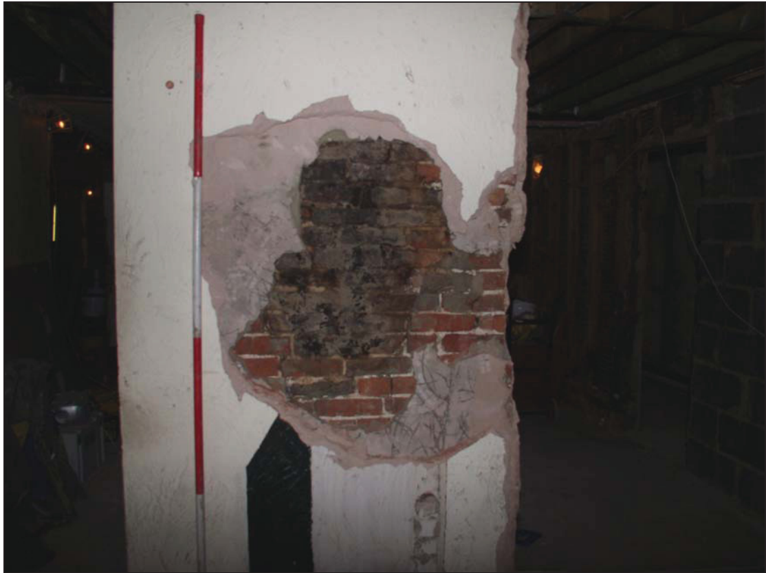
5 Eighteenth century brickwork of free-standing chimney stack plus sooted area marking position of flue, taken from the south (30)
