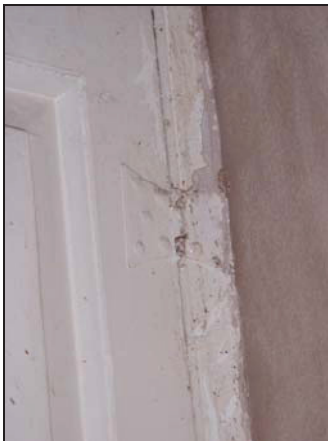
71 Butterfly hinge on cupboard door, first floor landing, principal range, taken from the north
