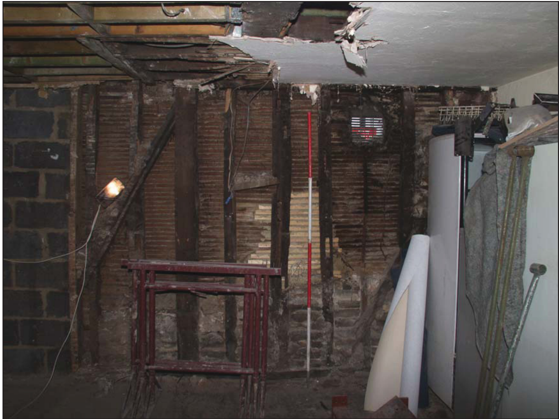
7 Primary braced framing on east wall of Room 2 utilising reused timbers, and bridging joist above, taken from the west (29)
