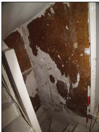
59 North wall of the stair tower showing plasterwork after removal of wallpaper, taken from the south-east
