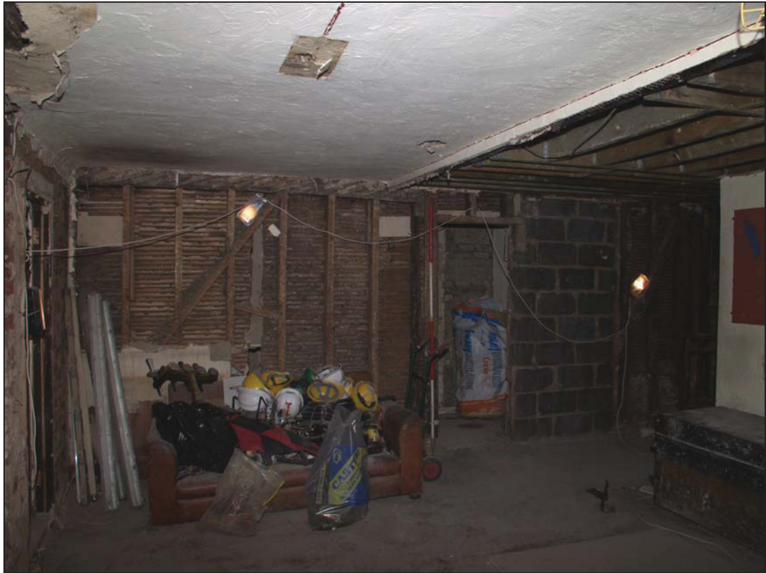
9 Twentieth century primary braced framing on east wall of Room 3, with original middle rail visible above, taken from the west (31)
