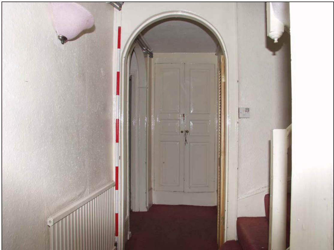
18 Eighteenth century archways and cupboard on first floor landing, principal range, taken from the north (15)
