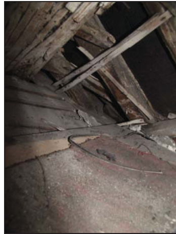
68 View into roof space at second floor level, taken from the north- east
