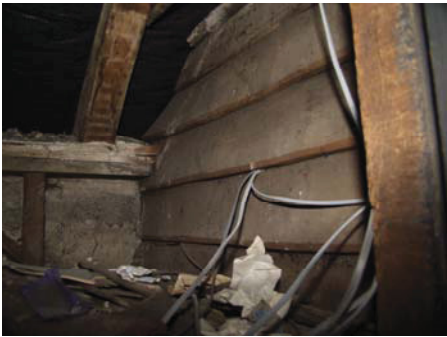
69 View into roof space at second floor level showing south side of stair tower, taken from the south- east
