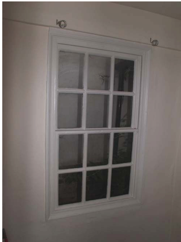
Plate 6 Early 18th century window on the north side of the stair, taken from the south-west (DP 28)
