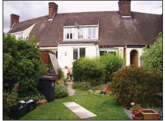
2 Rear of 2 Manor Cottages showing the new foundation trenches under excavation, looking north.
