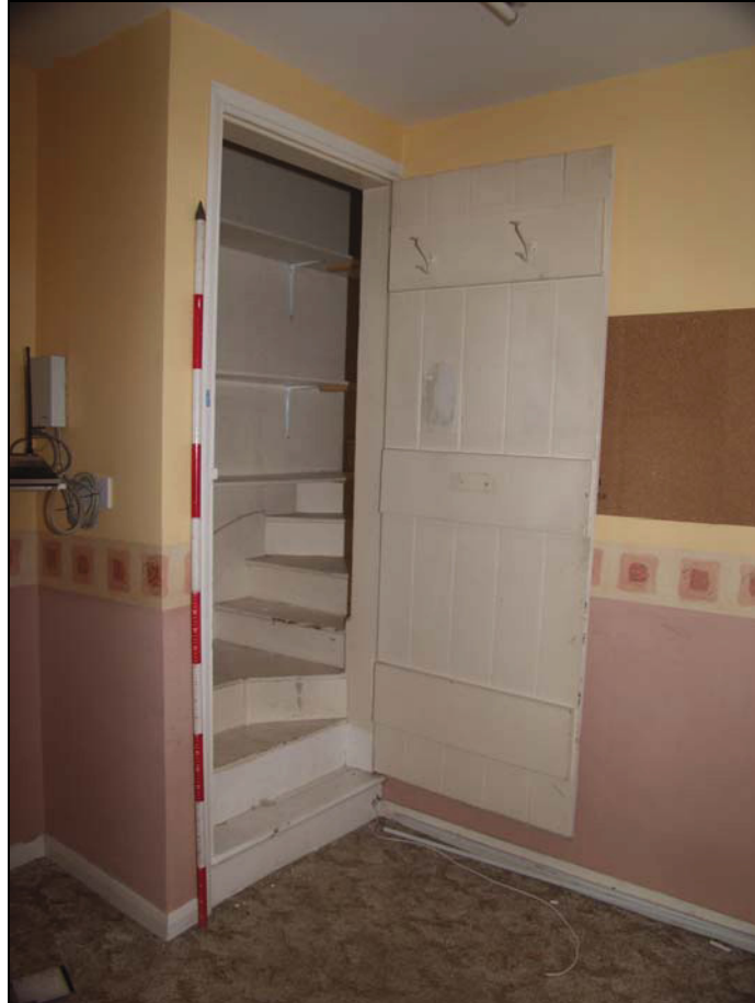
Plate 5 View of truncated stair in ground floor office, taken from the north-west (DP 12)
