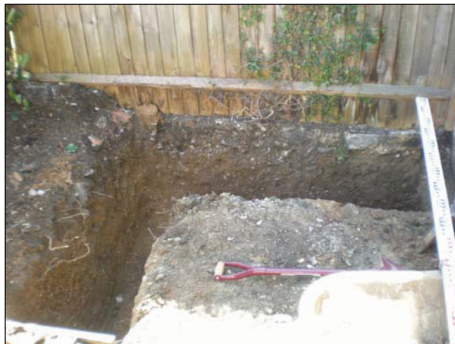
DP 3. Foundation trench to the rear of the house, SE corner. Taken from WNW.
