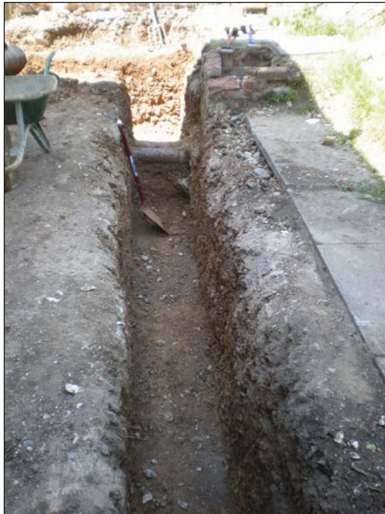
DP 8. W-E foundation trench to the rear of the house. Taken from ESE.
