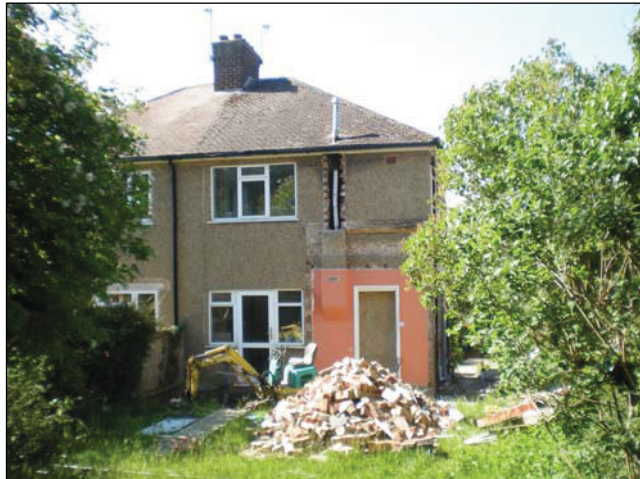
DP 2. Rear of the house with works on the site. Taken from NNW.
