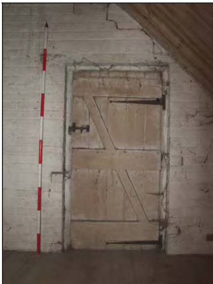
129 Rear side of the door between Rooms 1 and 2, Building 7: first floor, taken from the south
