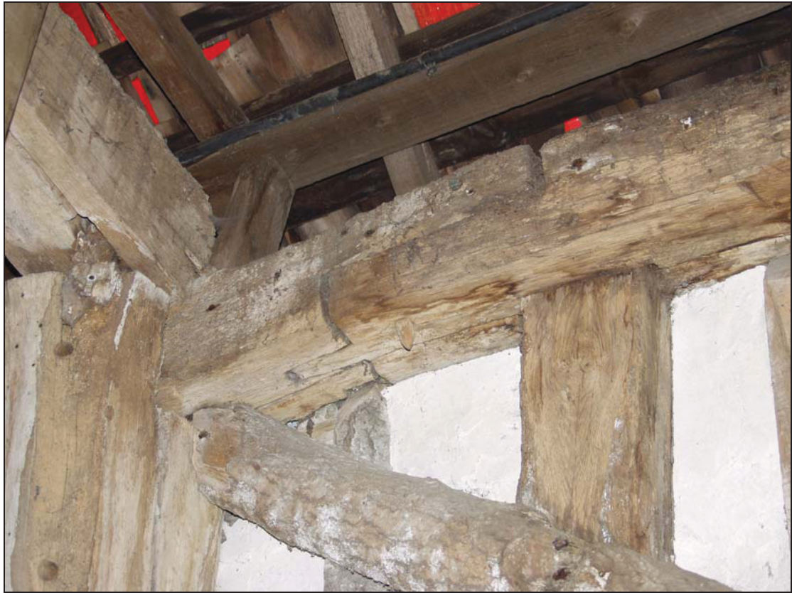
Plate 5 Detail of edge-halved and bladed scarf joint in the west wall-plate of Building 1, Bay 7, taken from the north-east (DP 85)
