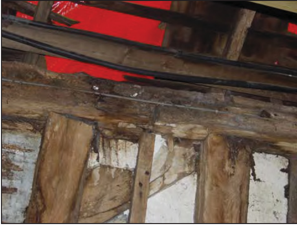
91 Scarf joint in the west wall-plate of Building 1, Bay 3, taken from the east
