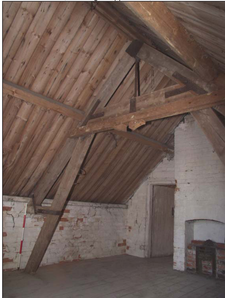
Plate 20 View of roof truss in Room 1, Building, taken from the north-east (DP 125)
