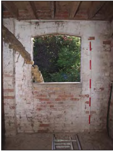
115 Window on the east wall of the stable, Building 7, taken from the west
