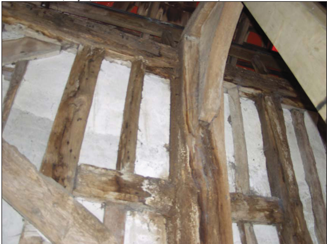
Plate 6 Detail of former window on the east wall of Bays 8 and 9 of Building 1, taken from the east (DP 84)
