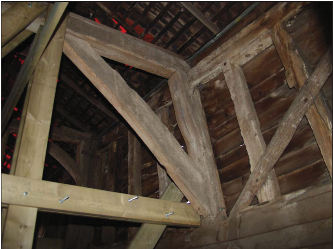
Plate 2 Detail of truss construction on the east side of Truss 6, Building 1, taken from south-west (DP 61)
