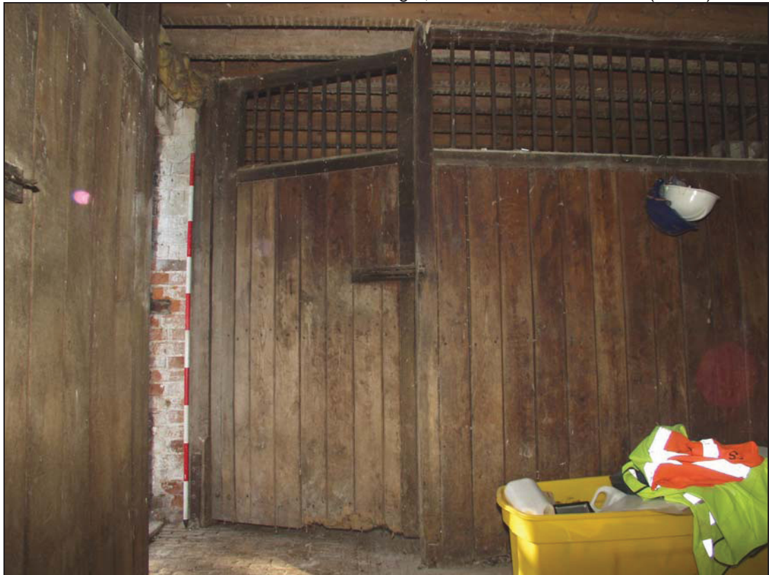
Plate 18 Partition and doorway to the south loosebox in the stable, Building 7, taken from the north (DP 113)
