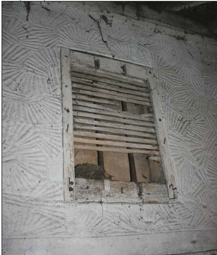
Plate 10 Detail of early window in the formerly external west wall of Building 2 from within the outshut, taken from the west (DP 141)
