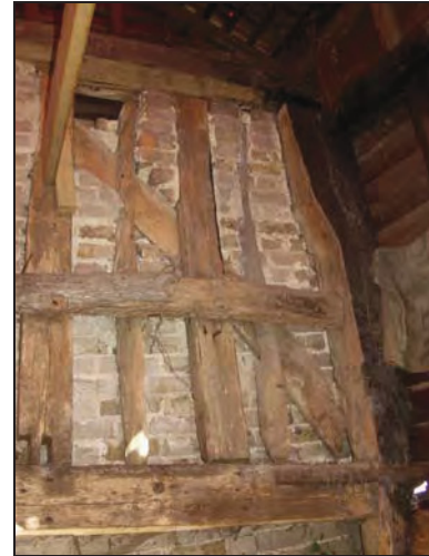
94 North gable of Building 1 showing external brace in the east register, taken from the south
