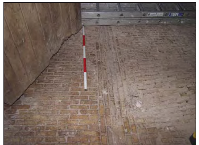
120 Detail of the floor in the stable showing the drain, Building 7, taken from the north
