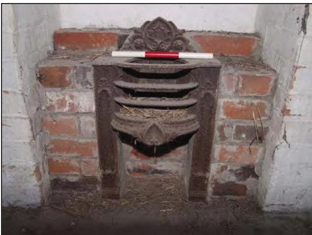
131 Detail of grate in the fireplace on the south side of Room 1, Building 7: upper floor, taken from the north
