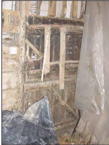
93 Door on the west side of Bay 1, Building 1, taken from the south-east
