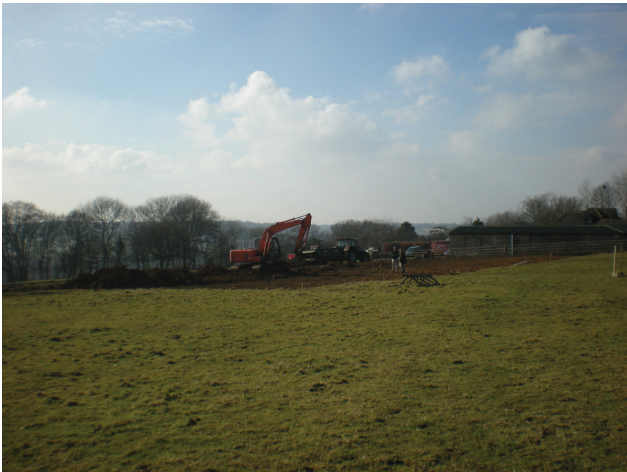
DP 1. Land at Hill House, Chalk Lane, Hyde Heath, Little Missenden, Buckinghamshire. View SW.
