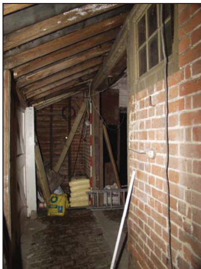
23 Formerly external east wall of south carriage house (Building 3), taken from the north-east
