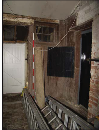
20 South-east corner of Building 3 showing wide vertical boarding, taken from the north-west
