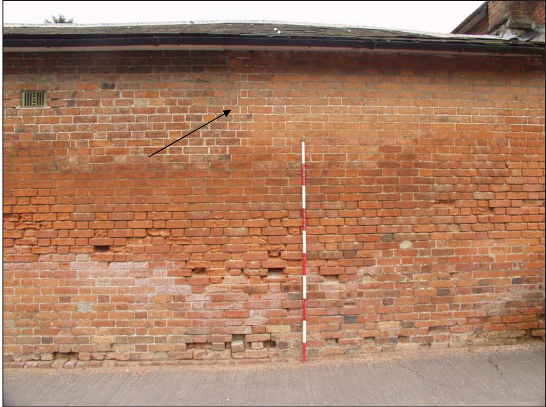
Plate 3 Line of queen closers (indicated) in the west wall (above level of the former garden wall) showing division between Buildings 3 and 4, taken from the west (40)
