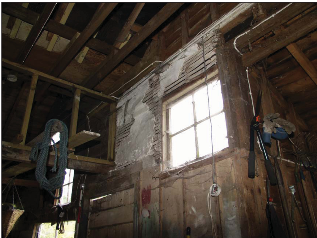
Plate 10 South wall of the central unit of Building 5, taken from the north-west (37)
