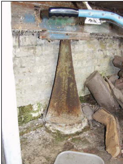
33 Detail of surviving stylobate in the east unit of Building 5 (north wall), taken from south-west
