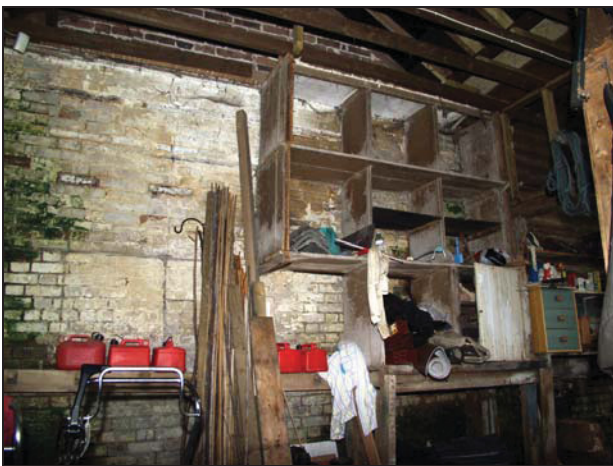
35 North wall of the central unit of Building 5, taken from the south
