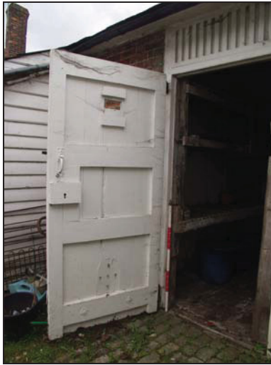
27 Rear side of door to storage unit (Building 4), taken from the north-east
