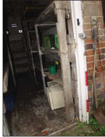
26 Detail of locking bar system to the storage unit (Building 4), taken from the south-east
