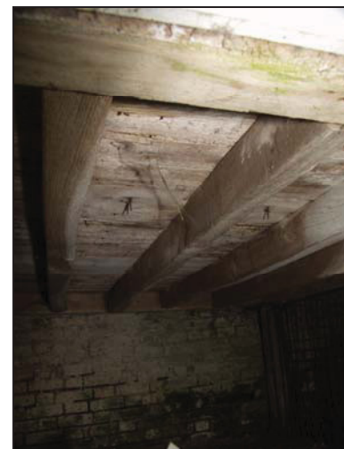
30 Detail of joists beneath granary (west end of Building 5), taken from the south
