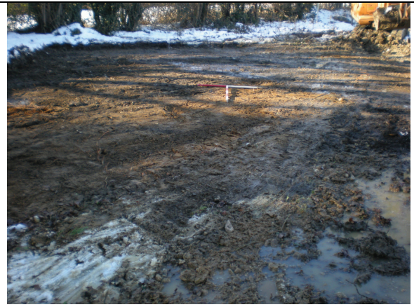
DP2 Ground reduction in the area west of the entrance (view north-west)
