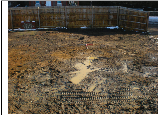
DP1 Ground reduction in the area east of the entrance (view south)
