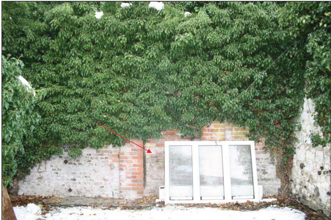
Plate 1 Obscured view of the retaining wall showing blocked doorway (indicated), taken from the west (DP 04)
