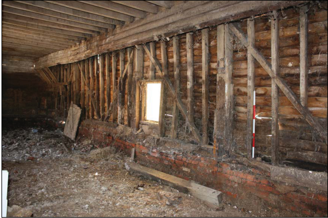
Plate 5 South wall of the barn (after stripping out), taken from the north-west (DP 45)
