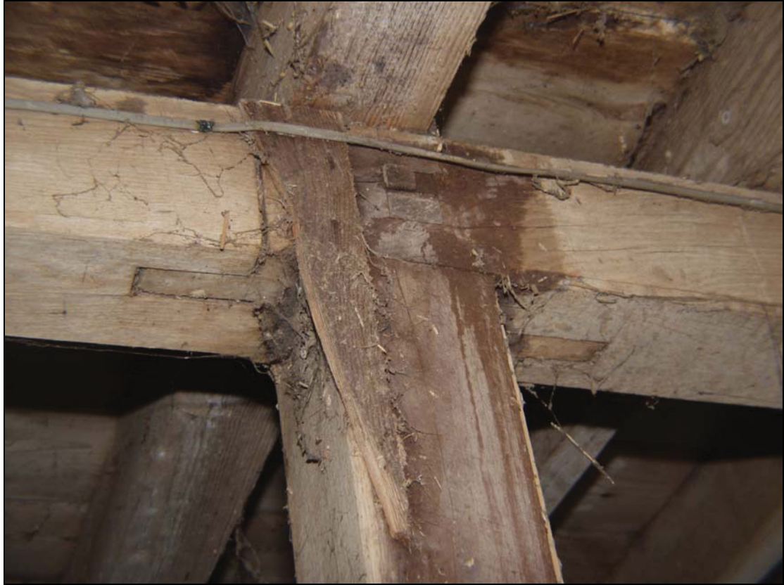
Plate 3 Detail of scarf joint in bridging joist in the barn, taken from the north-east (DP 11)
