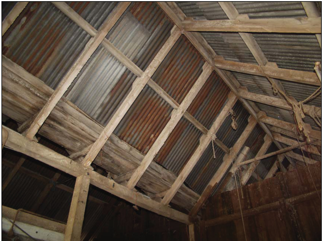
Plate 2 Detail showing roof construction of the milling barn, taken from the north (32)
