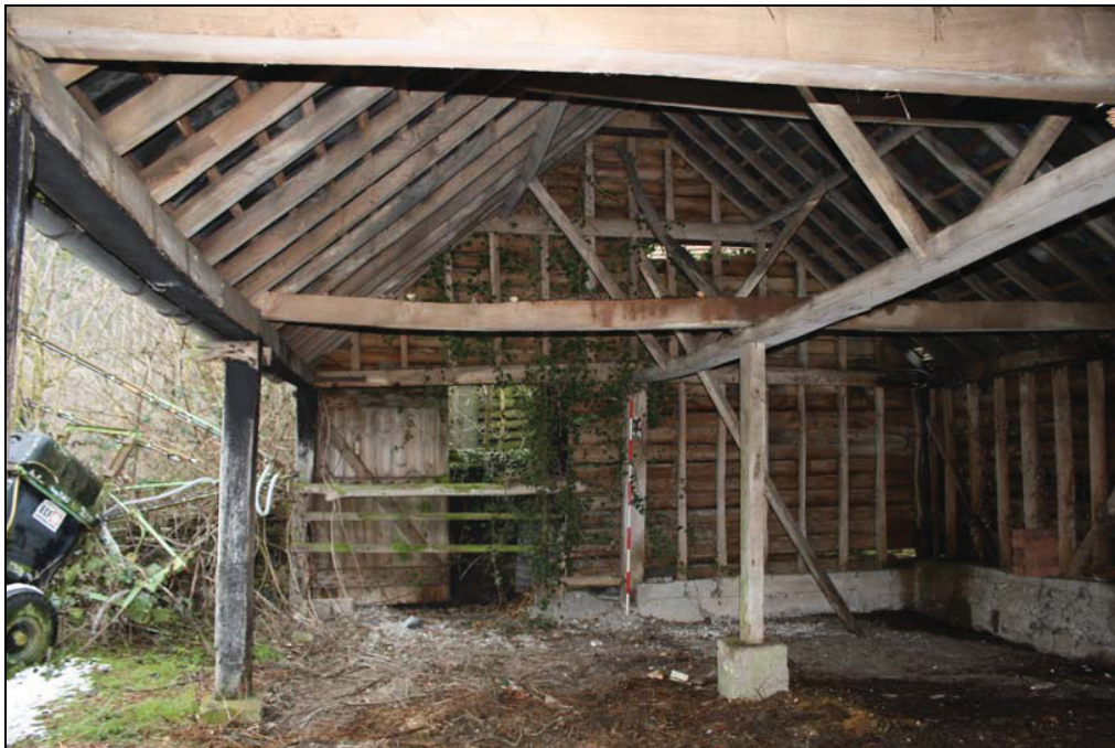
Plate 21 The cart shed, internal, northern gable end, taken from the south (DP 9)
