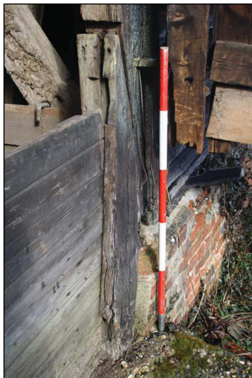
Plate 12 The barn, threshing leap, eastern jamb of main entrance, taken from the south-west (DP 40)
