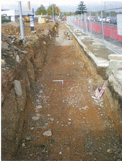
DP 3. Service trench along the N edge of the site. View WSW.
