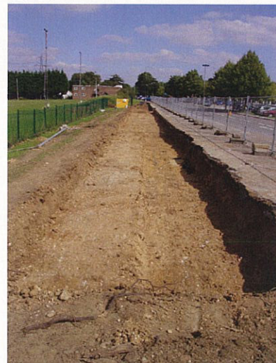
DP 4. Service trench to the N of the access road. View ENE.
