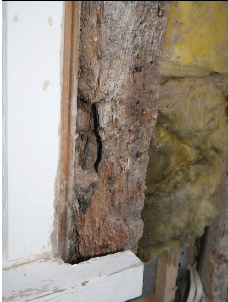
Plate 5 Mortise for the sill piece of an original window in the west bay of the upper floor, taken from the south-west (DP 40)
