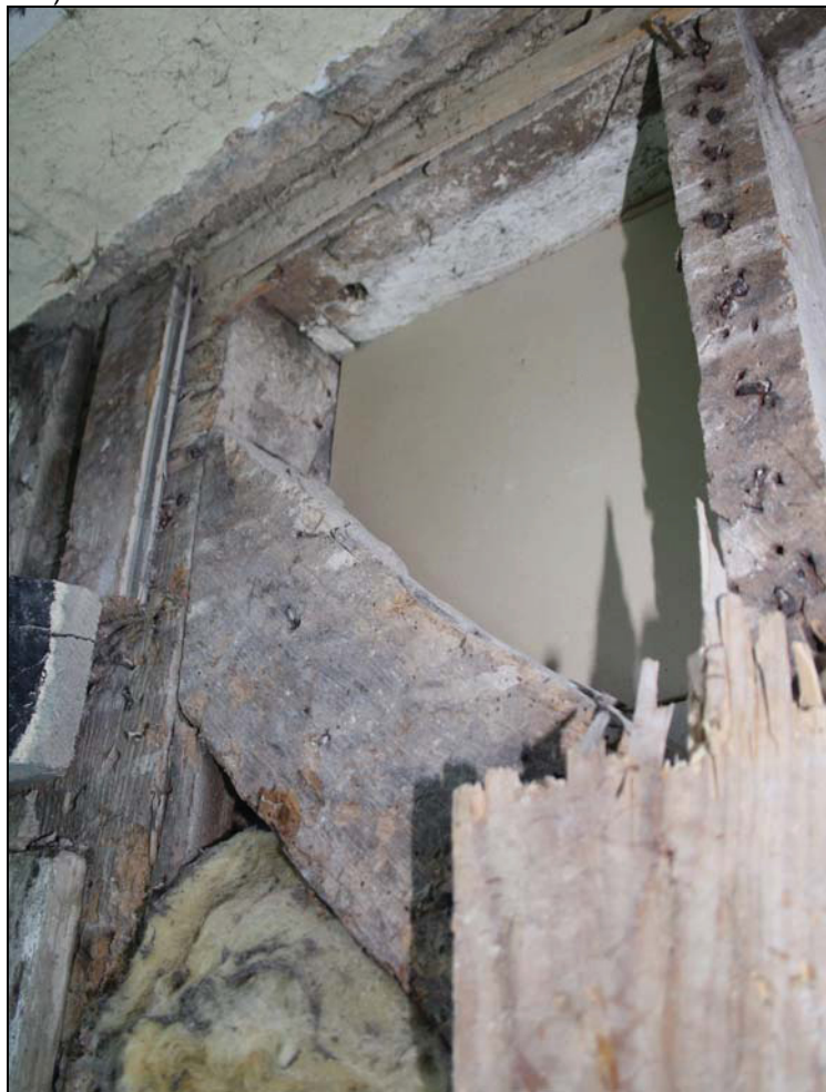
Plate 4 Detail of later primary-brace and redundant wattle hole in the wall-plate of the west bay, taken from the south-east (DP 39)
