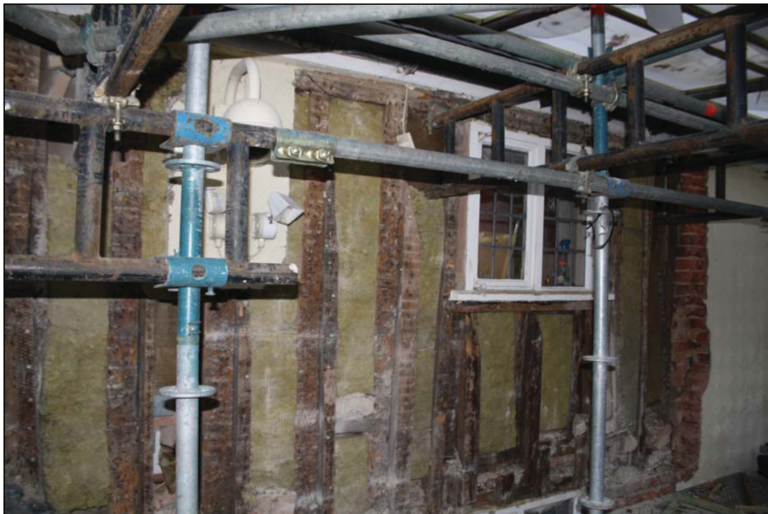
Plate 6 Timber-framing of the east bay at upper level, taken from the south-west (DP 47)
