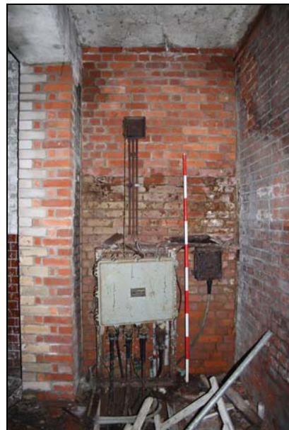
12 Switching gear, taken from the west
