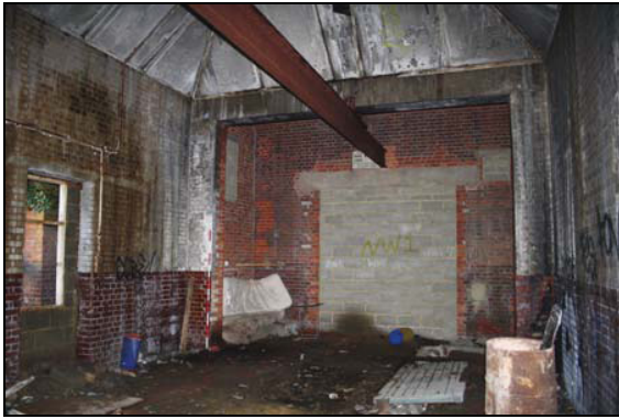
7 Engine room, taken from the south-east
