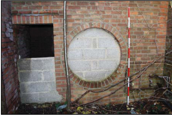
21 Blocked apertures from fuel tank storage area into transformer chamber, taken from the south
