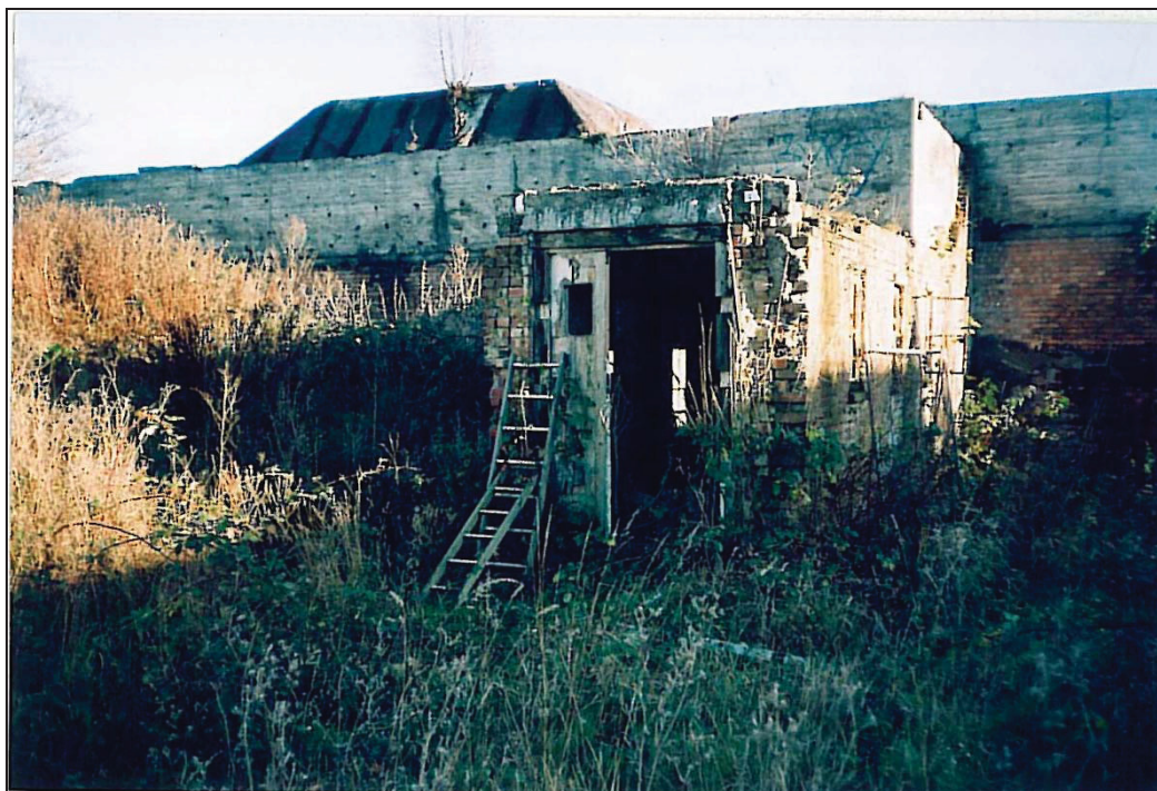
2009: The exit from the Site Quarters Annex, which led to a walkway/corridor to the main Sick Quarters building.
