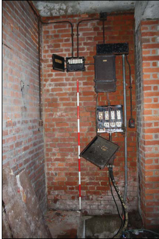
Plate 5 Switching gear, taken from the east (DP 11)
