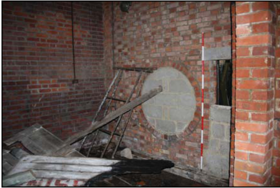
15 Transformer chamber, taken from the north-west
