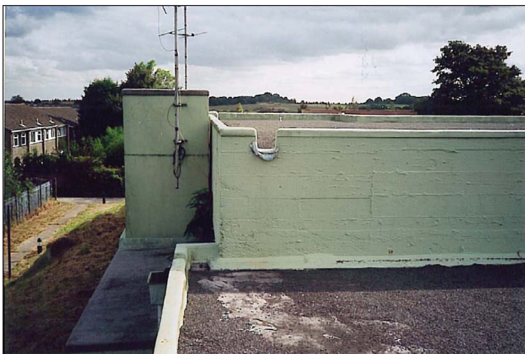
2002: The roof of the Operations Block, converted to an Emergency Planning Centre in 1989. Note the air intake/filtration unit on the left.
