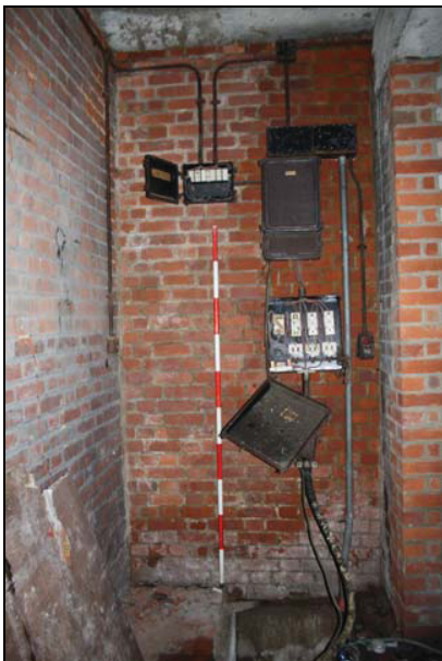
11 Switching gear, taken from the east
