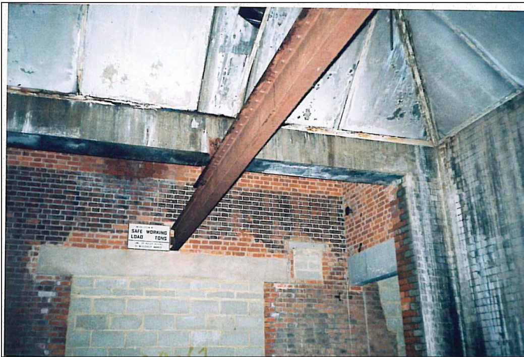
2009: Inside the expanded engine room a crane rail was installed. This allowed the heavy diesel engines to be lifted in and out through the new entrance.
