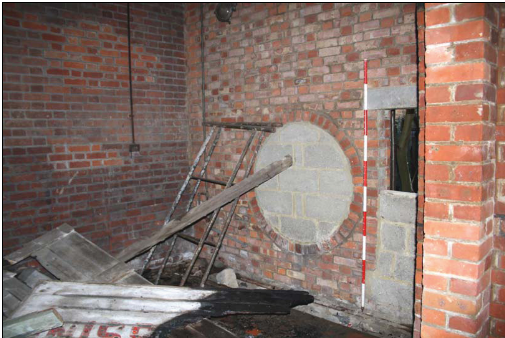
Plate 6 Transformer chamber, taken from the north-west (DP 15)
