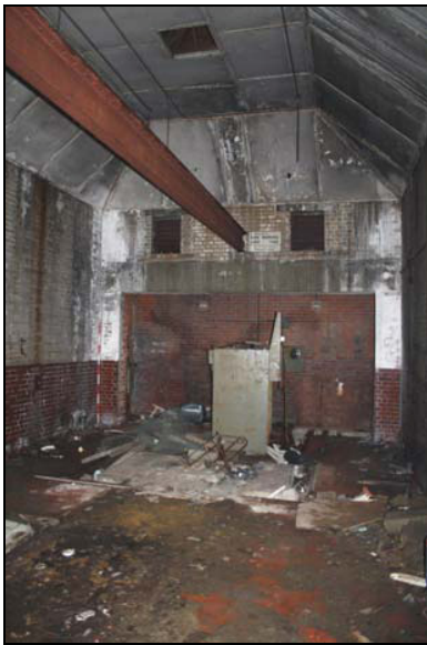
9 Engine room and machinery, taken from the north-west
