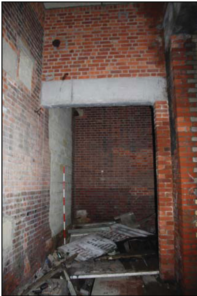
17 Transformer chamber, taken from the west
