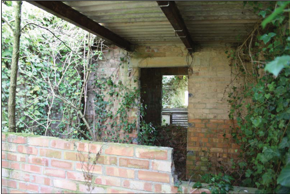
Plate 9 South-west range adjacent to the gymnasium, interior, taken from the west (DP 44)
