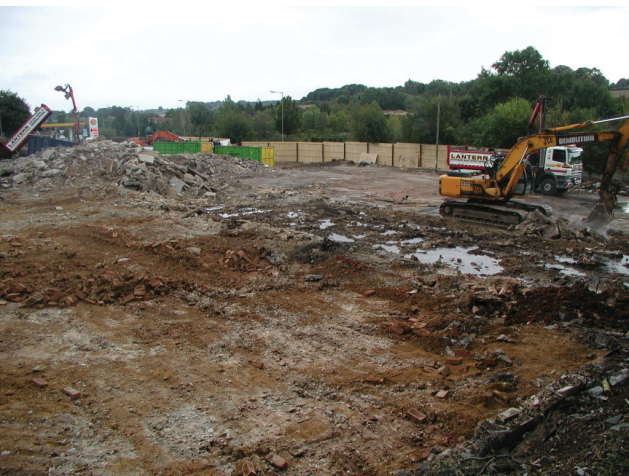
DP 11. Removal of concrete floor of the warehouse after its demolition. View SE.
