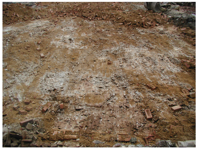
DP 12. The S part of the warehouse after removal of concrete floor. View ESE.
