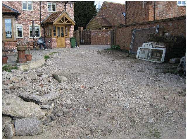
DP 10. E part of the property prepared for a new yard and access road layout. View NE.
