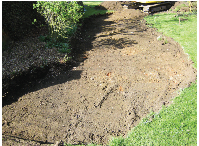
DP 4. Ground reduction for a new access road, part E. View WNW.
