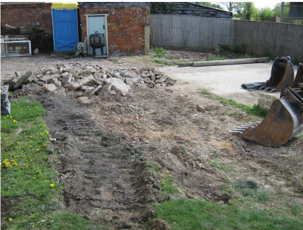
DP 9. SE part of the property prepared for a new yard layout. View ENE.
