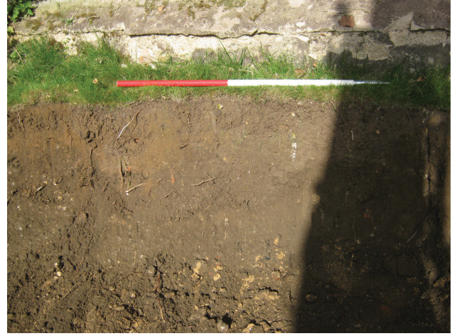
DP 8. Ground reduction for a new access road, part E. Sample section. View NW.
