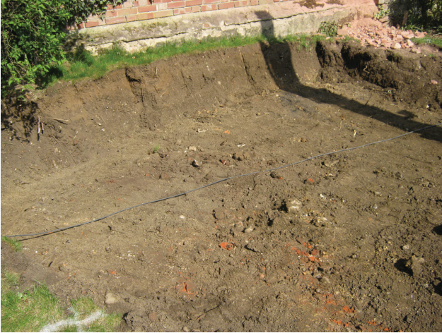
DP 7. Ground reduction for a new access road, part W. View N.
