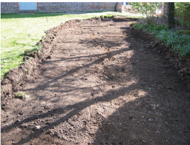
DP 5. Ground reduction for a new access road, part E. View ENE.
