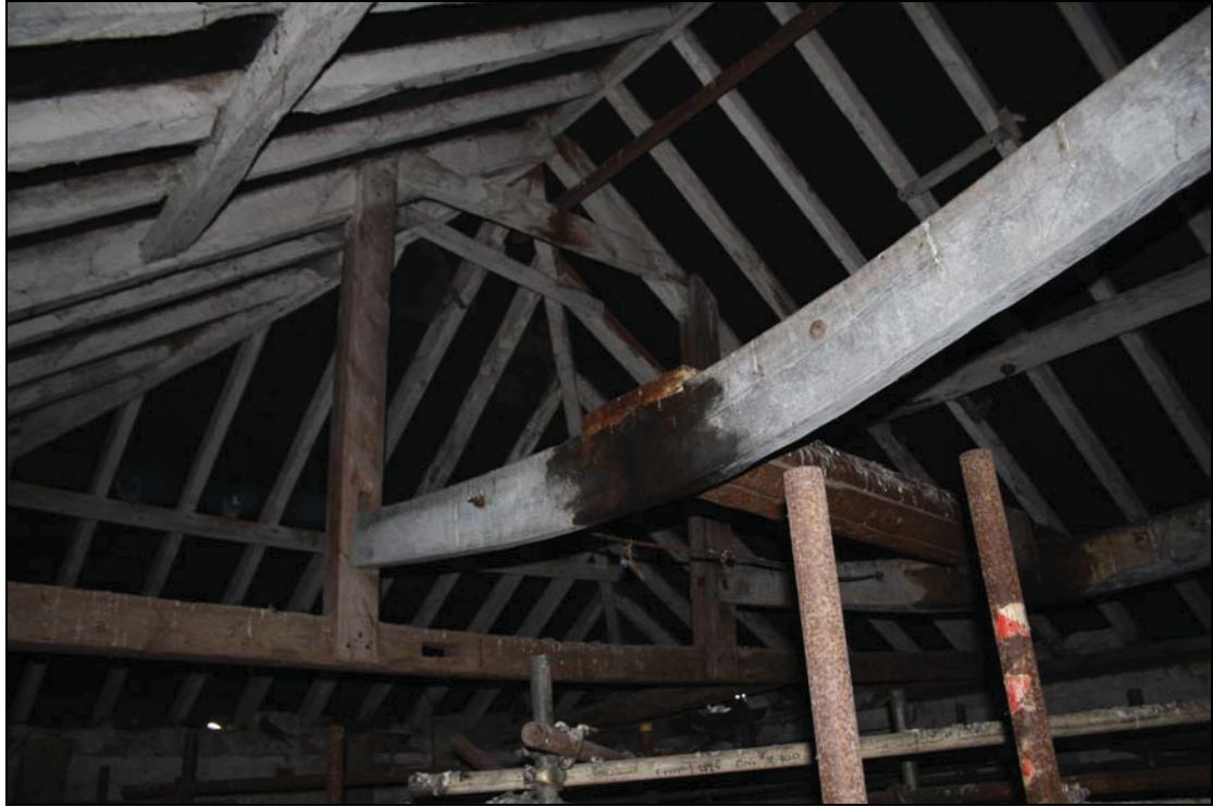
Plate 9 Queen post roof construction with cambered hanging joists, taken from the north-east (DP16)
