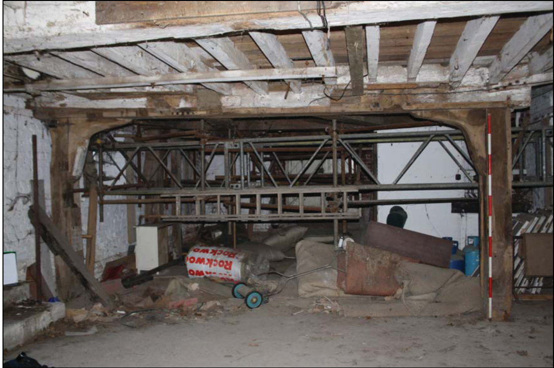
Plate 5 Ground floor oak timber framing to house mill machinery, taken from the north-east (DP 22)
