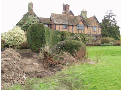
DP1. Location of trench in relation to the NW façade of Cheddington Manor, looking S (01/04/2010)
