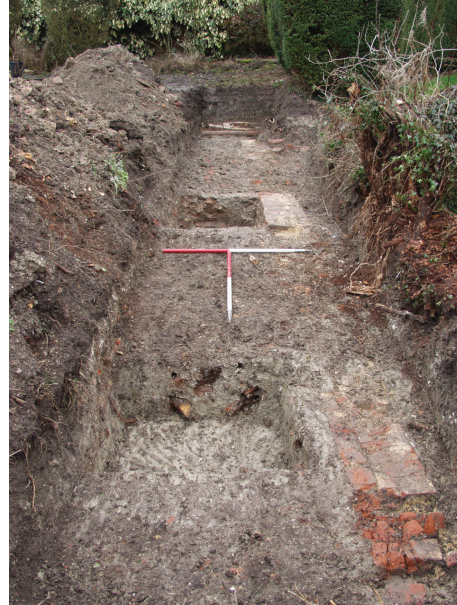
DP2. Post-excavation view of trench, wall M1004 running the length of the trench, looking SE (01/04/2010)
