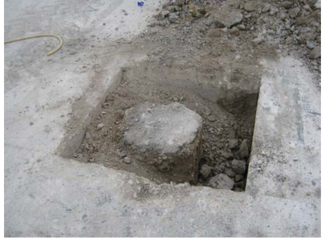
DP 8. Trench for a pile in central part of the site. View SSE.
