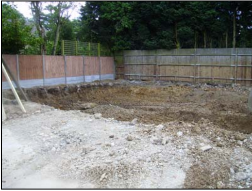
30 Footprint of proposed office suite with cement surface in foreground. Looking S
