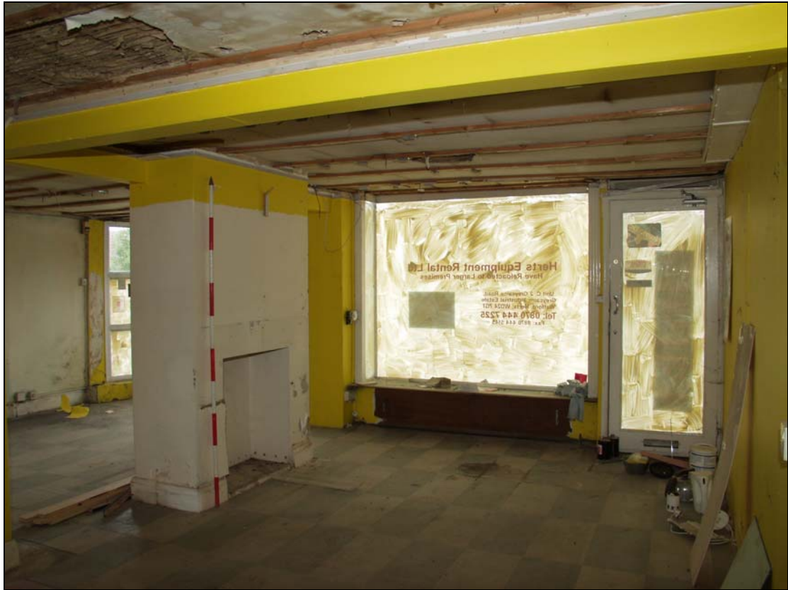
Plate 7 East side of Room 6 showing free-standing chimneystack (No. 195), taken from the south (DP 21)
