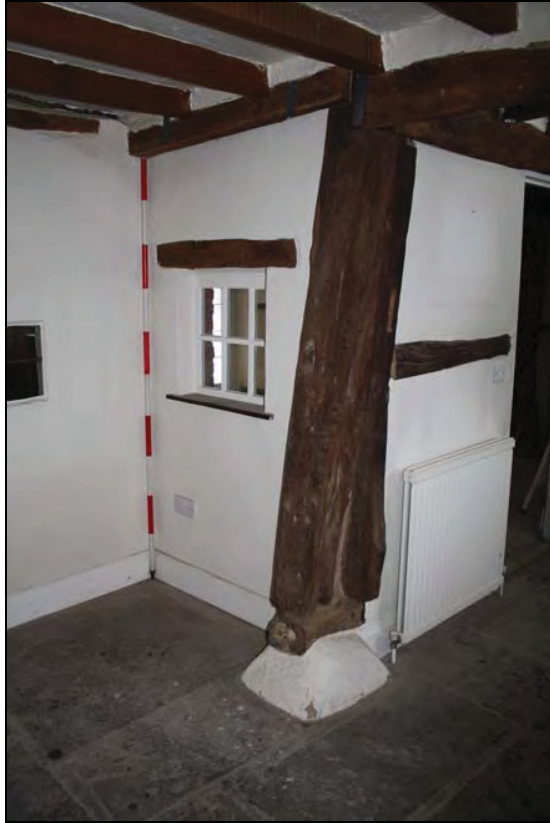
Plate 3 Entrance lobby (Room 1) and original corner post, taken from the west (DP 10)
