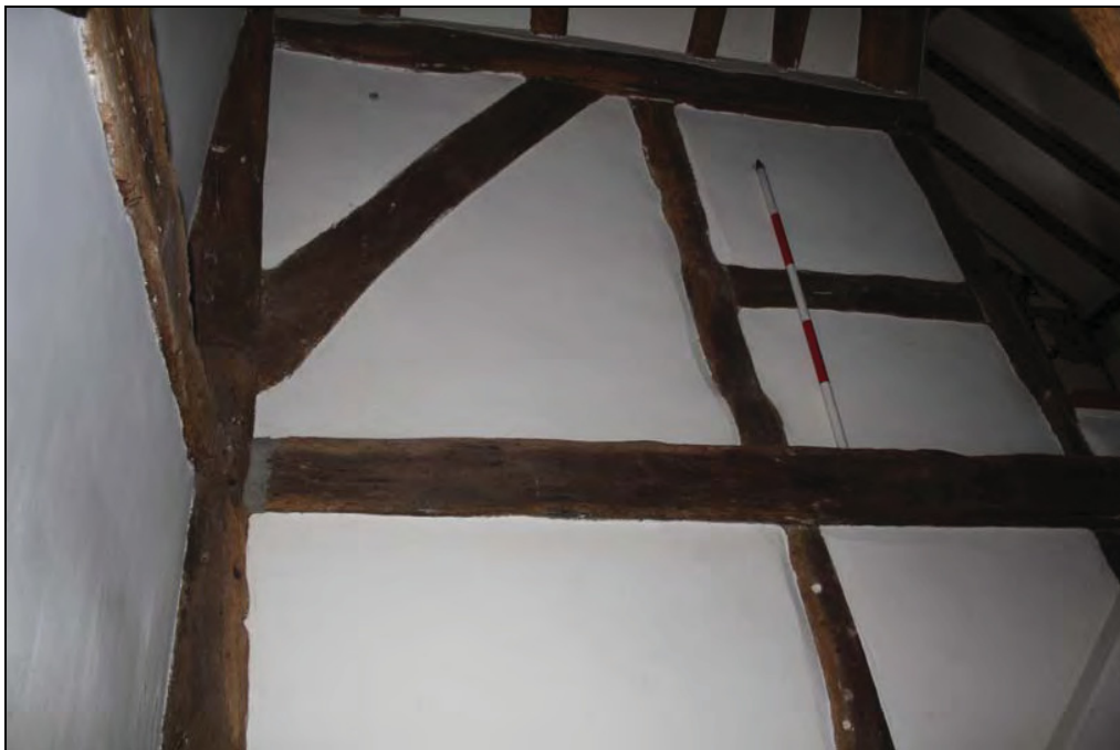
Plate 9 Original external wall with blocked window (Room 9), taken from the north-east (DP 33)
